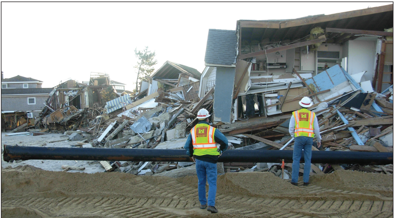
Houses devastated by Hurricane Sandy in Mantoloking, NJ on November 26, 2012
