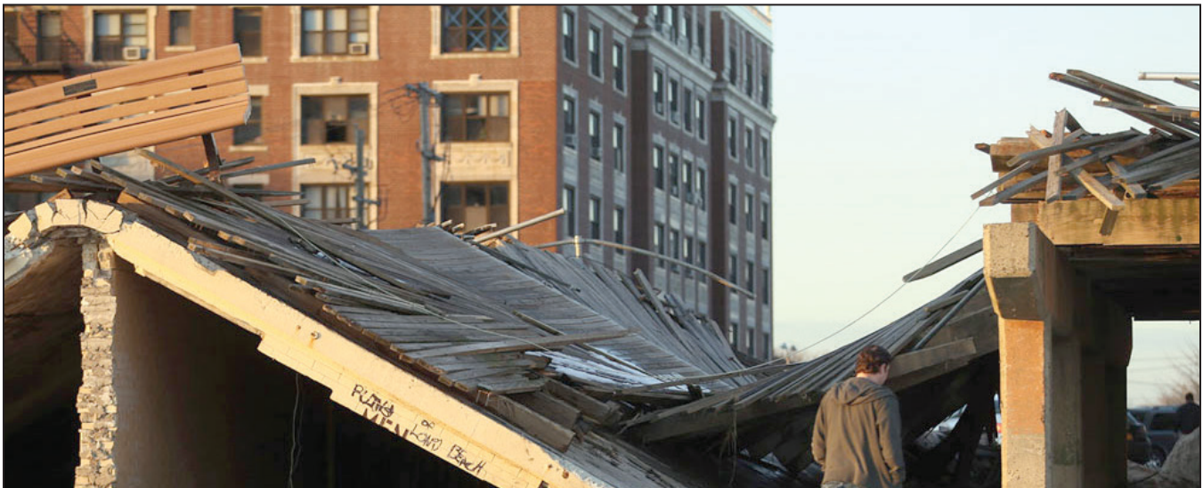
A section of boardwalk at the base of Lincoln Boulevard destroyed during Hurricane Sandy in Long Beach, NY
