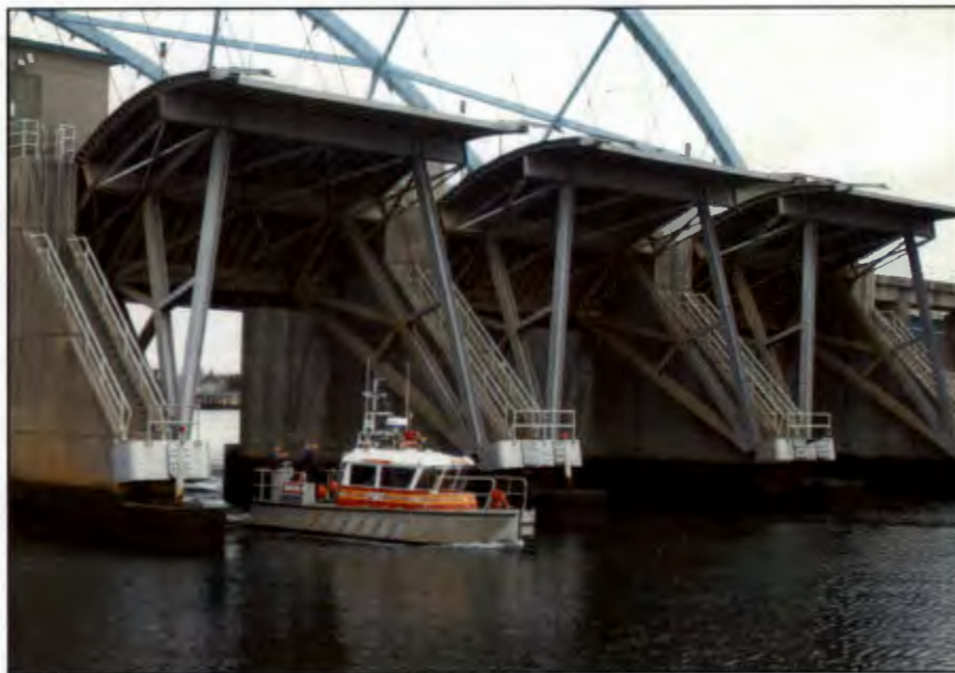
Figure D-5: Navigation Gates at the Fox Point Hurricane Barrier, Providence, RI
