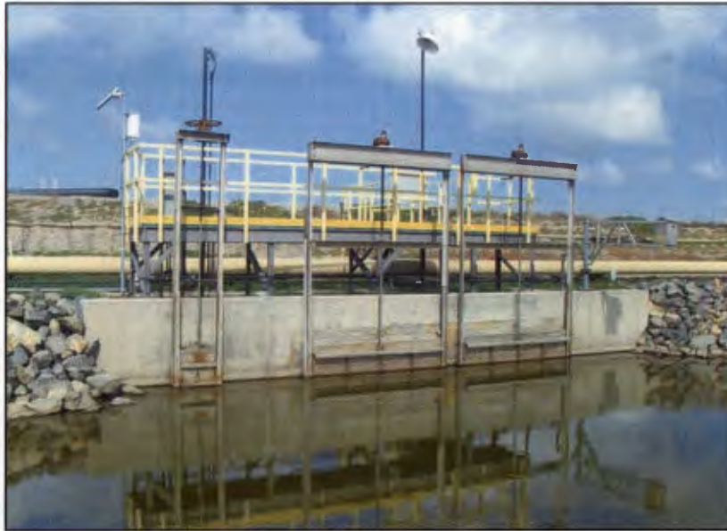
Figure D-10: Tide Gate at the Bolsa Chica Wetlands Restoration Project, CA
