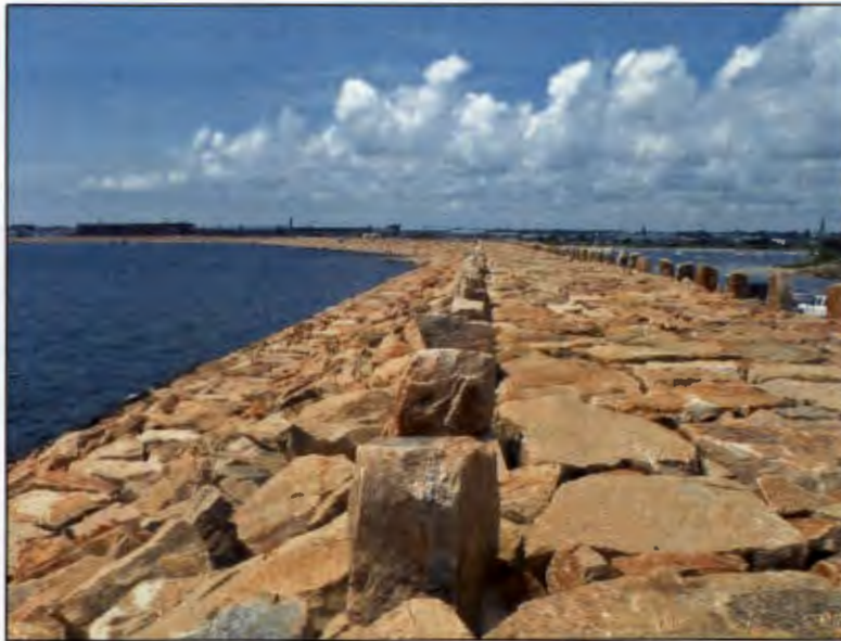
Figure D-2: Dike constructed as part of the New Bedford Hurricane Barrier, MA
