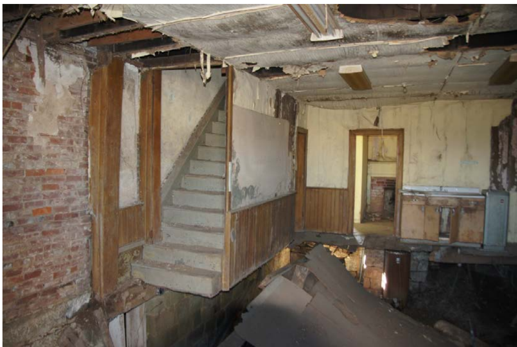
Photo 50. Room 8 – First floor of frame house showing collapsed floor and stairway to second floor, looking southwest.
