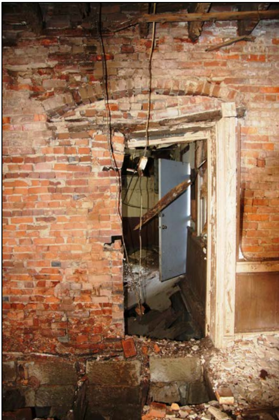
Photo 33. Room 3 – Juncture of brick house and frame section, showing partially in-filled door opening with relieving arch, rear/north wall.
