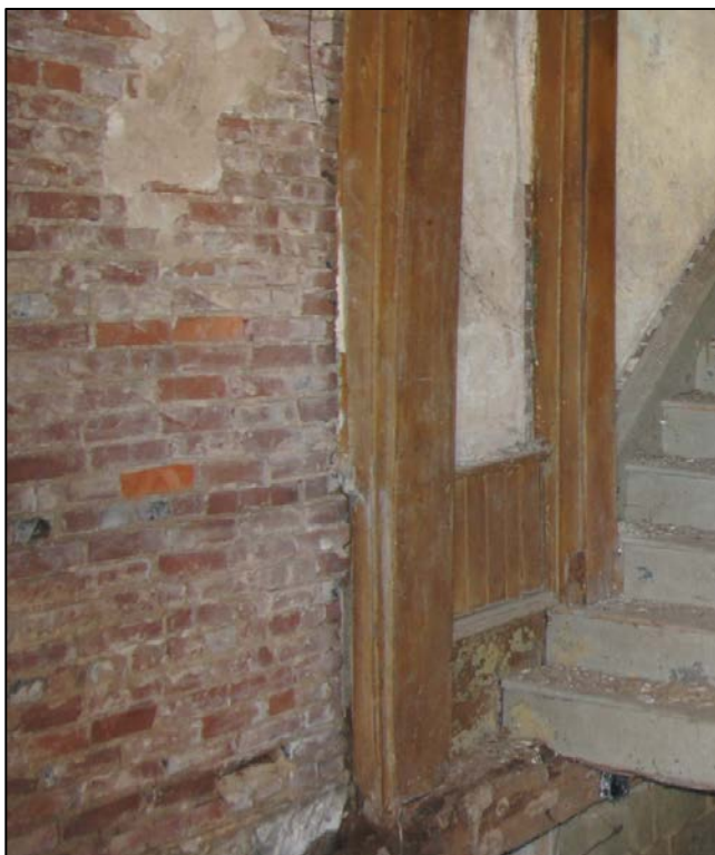
Photo 49. Room 8 – Detail, rear wall of the brick house, first floor, looking southwest. The mortar joints of this wall are struck and appear similar in profile, materials, and execution as joints on other exterior elevations of the house.
