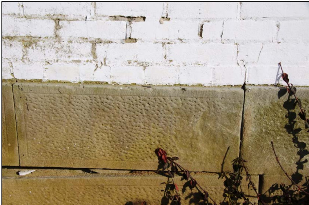
Photo 18. Original foundation, west elevation. Sandstone cap blocks exhibit bush hammered finish with chiseled margins.
