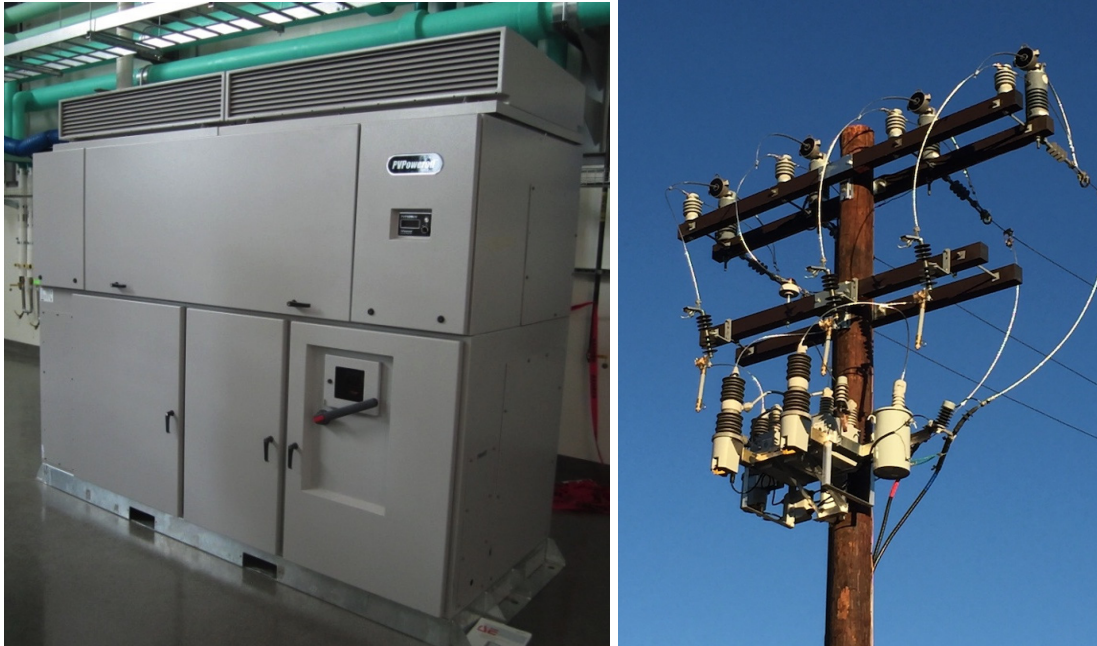
Figure 67. Power hardware installed at NREL (500TX and capacitor bank)
