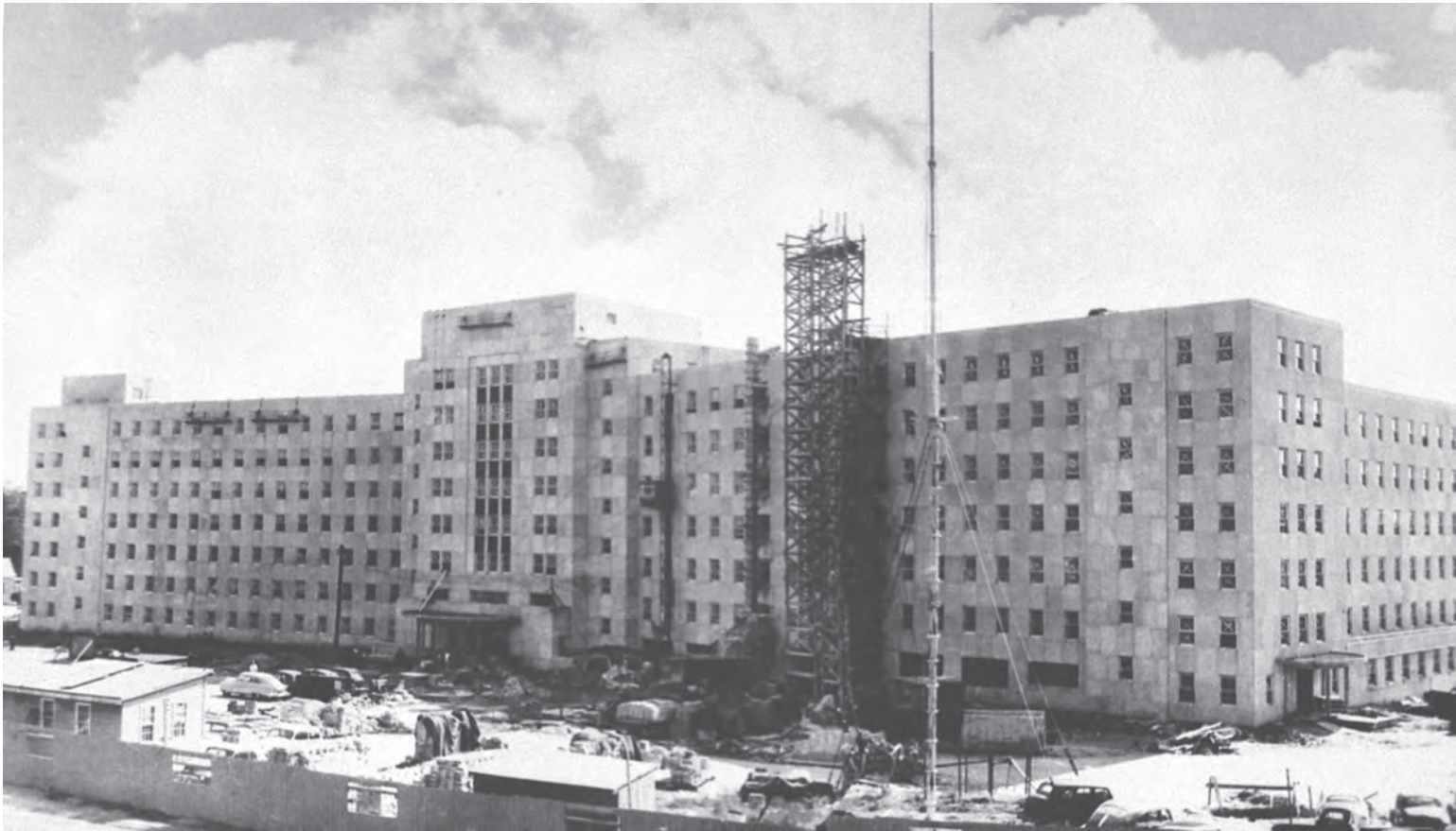
The 850-bed residence hall under construction at the U.S. Soldiers' Home, 1952, was named for Winfield Scott, who was instrumental in the establishment of the Soldiers' Home in 1851. Office of History, Corps of Engineers
