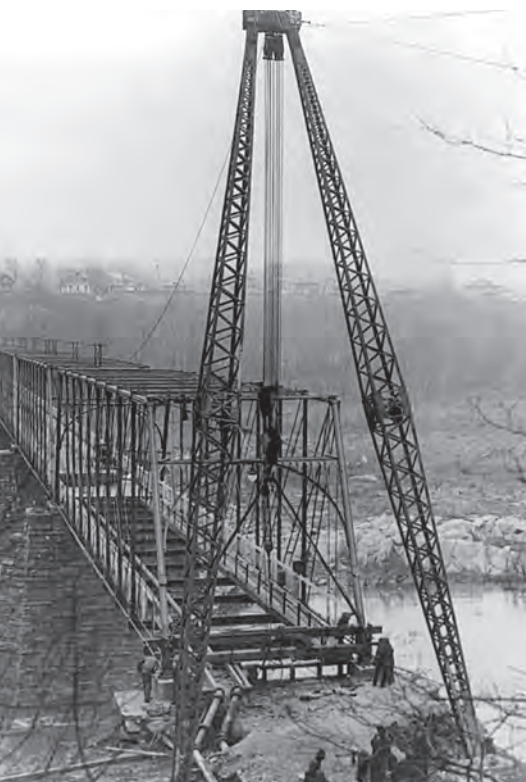
Chain Bridge undergoing repairs, 1928. One end of the wrought-iron bridge built by Babcock in 1874 was lifted to repair one of its piers.
