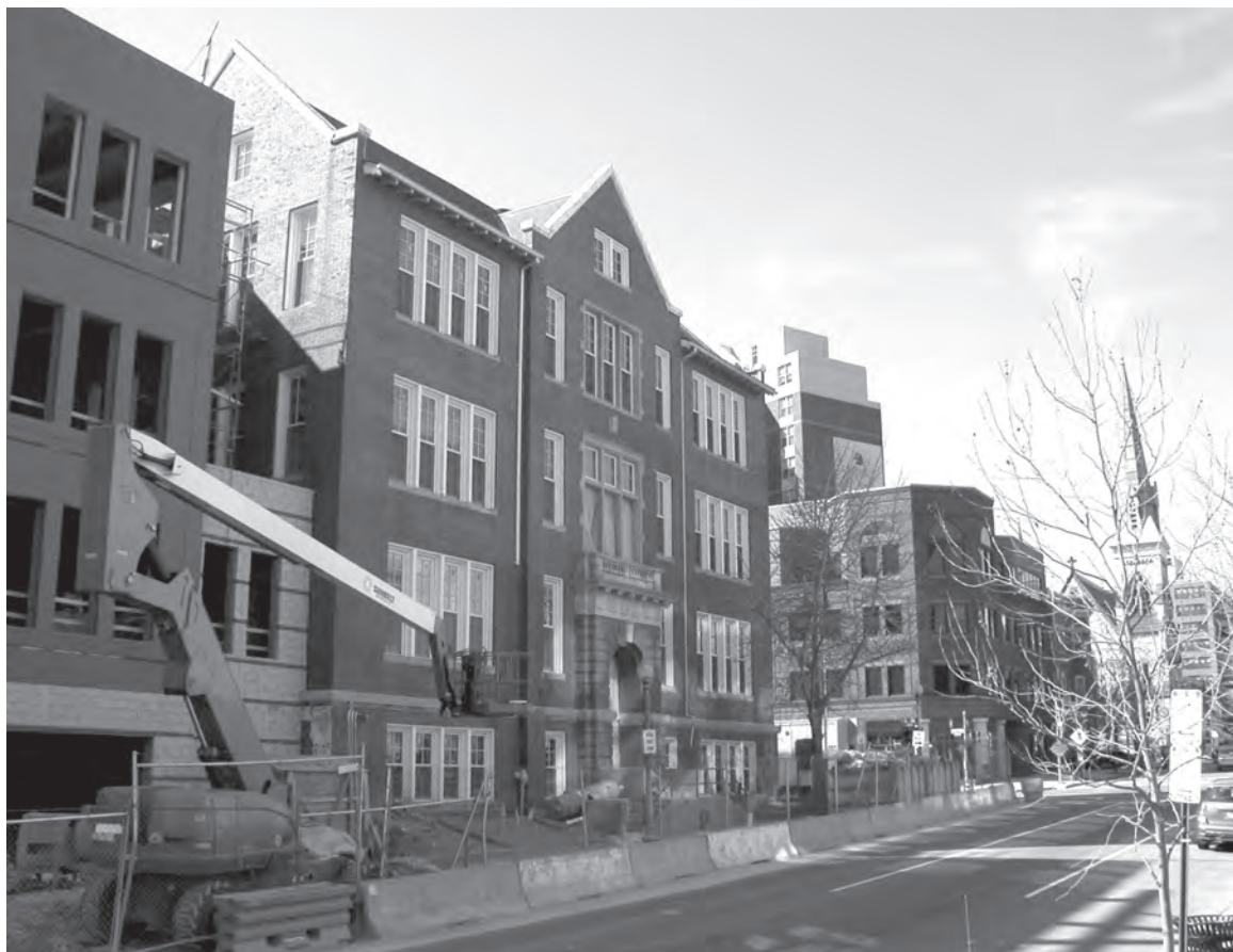
The Corps has made extensive repairs and built additions to the Thomson Elementary School in downtown Washington at 12th and L Streets, NW, which was scheduled to reopen for the 2005–06 school year. Photograph by Darren Santos
