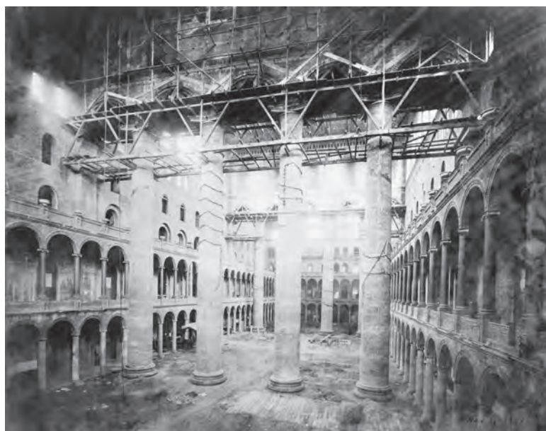
Pension Building under construction showing the massive brick central columns and the rows of columns on the first and second floors, November 1885
