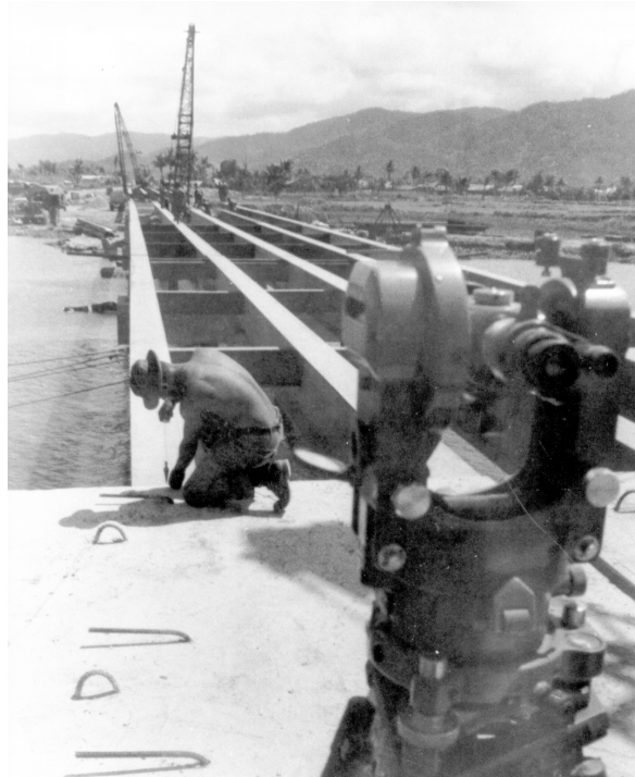
The 577th Engineer Battalion (Construction) built the Ban Thach River bridge from pre-cast elements in 1968.
