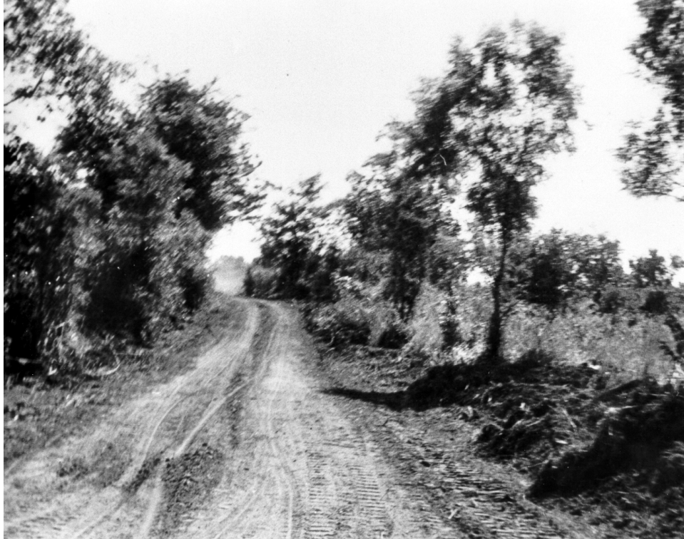
In August 1962 the 20th Engineer Group of the Army of the Republic of Vietnam was opening a road from Cheo Reo to Cung Son.
