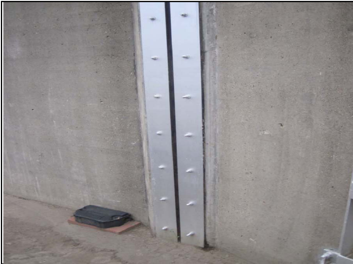
Figure 5: Alternative external waterstop on riverside of Newport, KY floodwall
