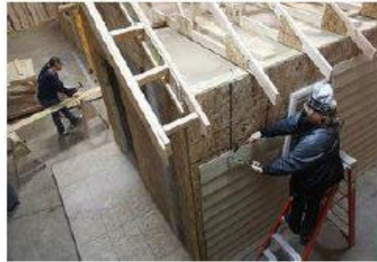
Angela Porter, 46, of St. Paul, hammered the nails out of the boards as she and her classmates deconstructed a house.
