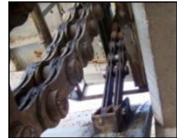
Failing gate hoist chains at Lock and Dam 25 – critical backlog repairs
