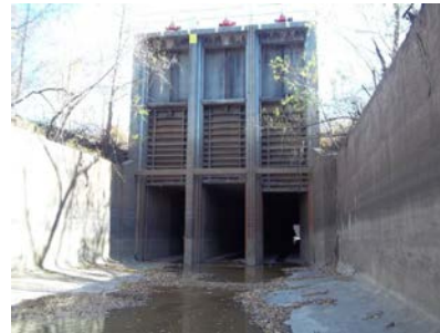
Pump Station Closure Gates
