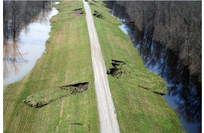
Typical Alton-Gale Levee Slides (2008 Flood)
