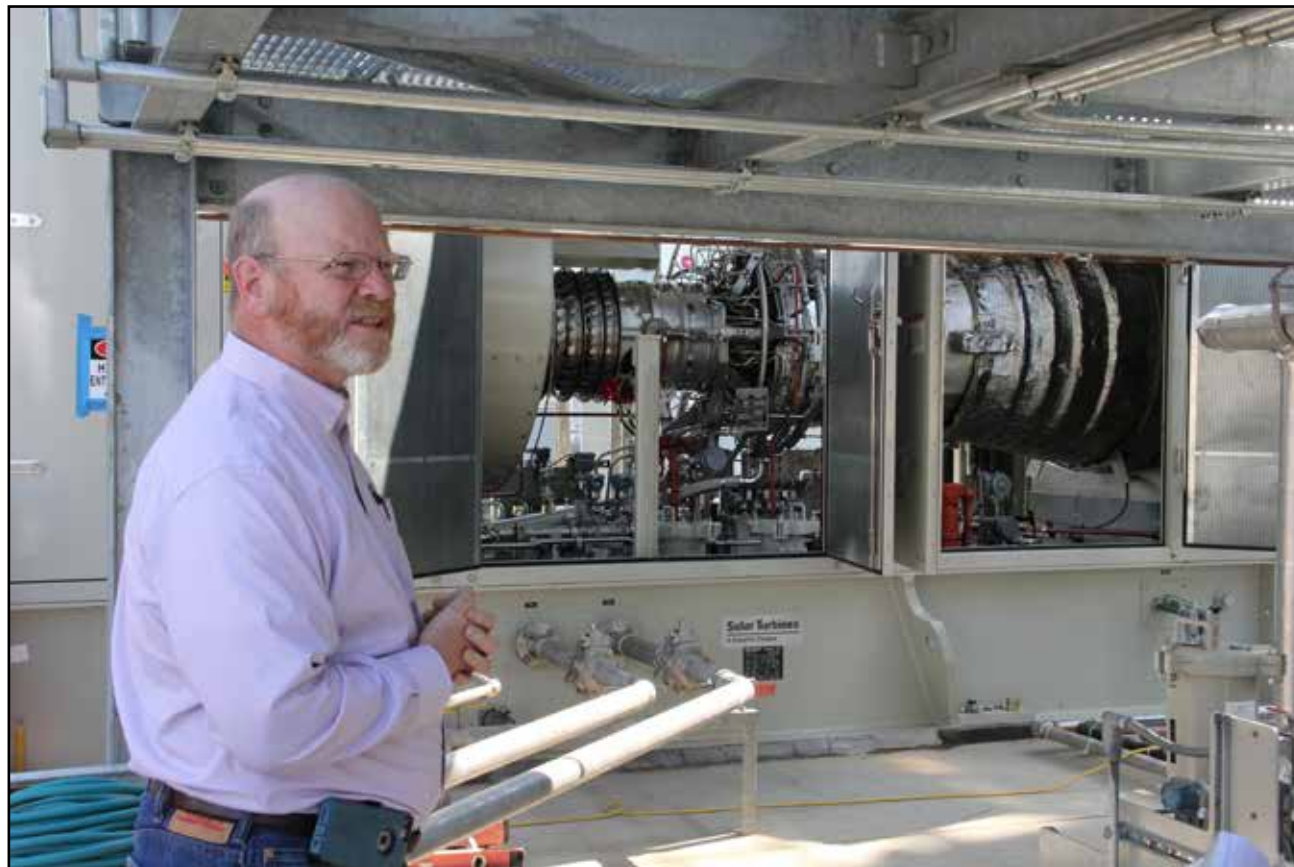
James Wyant, a contractor with Compass Commissioning and Design, provides a tour of the new Combined Heat and Power Plant at Aberdeen Proving Ground, Maryland, highlighting its features and improved efficiencies during the plant's "chain-cutting" ceremony July 19, 2016. The emerging technology will generate high-quality electricity and steam for the Edgewood Area of APG, saving the Army $4.4 million annually. (Photos by Molly Blosser)
