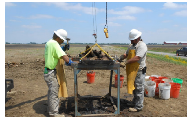
Contractors use the Thermal Flash Unit, which processes the remaining metal to remove any particles of white phosphorous. (Courtesy photo)
