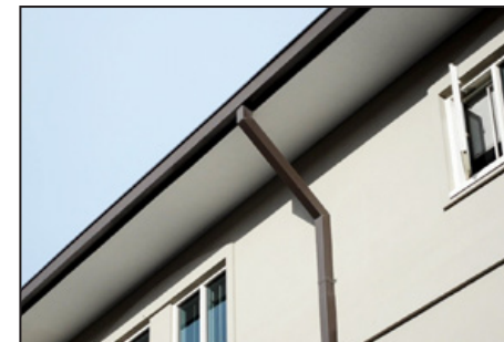
Water that will ultimately be used in toilets will not be pulled from the local water supply, but instead the building will collect it by recycling rainwater from the roof.
