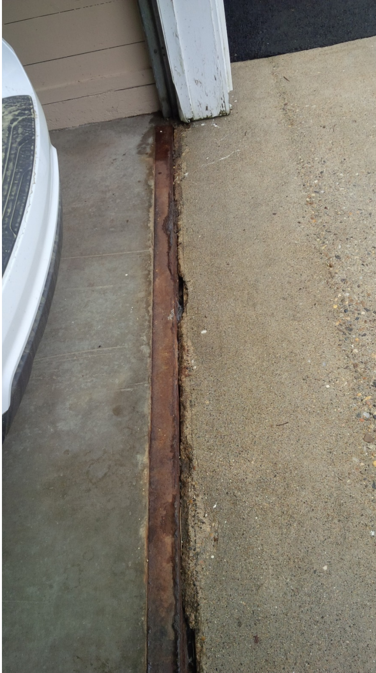
Informational Photo Number 6: Otter Brook Lake – Current condition of apron
