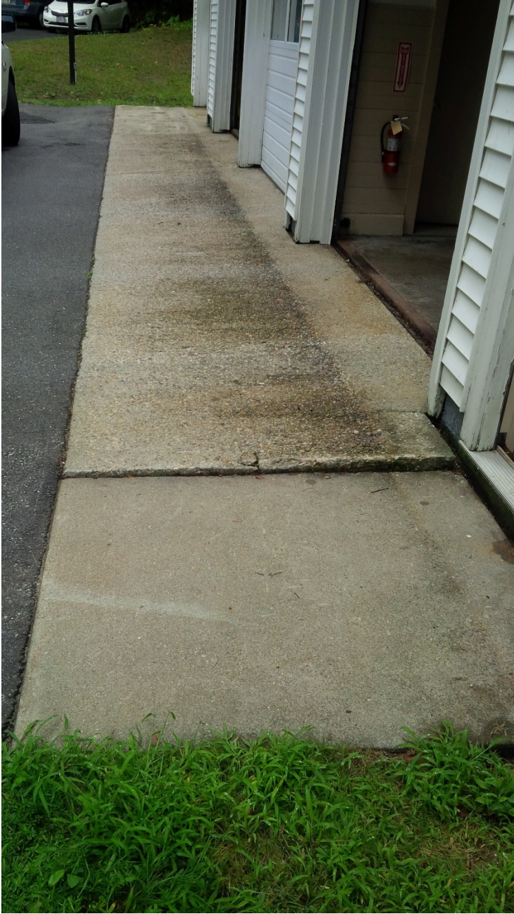
Informational Photo Number 2: Surry Mountain Lake – Current condition of apron
