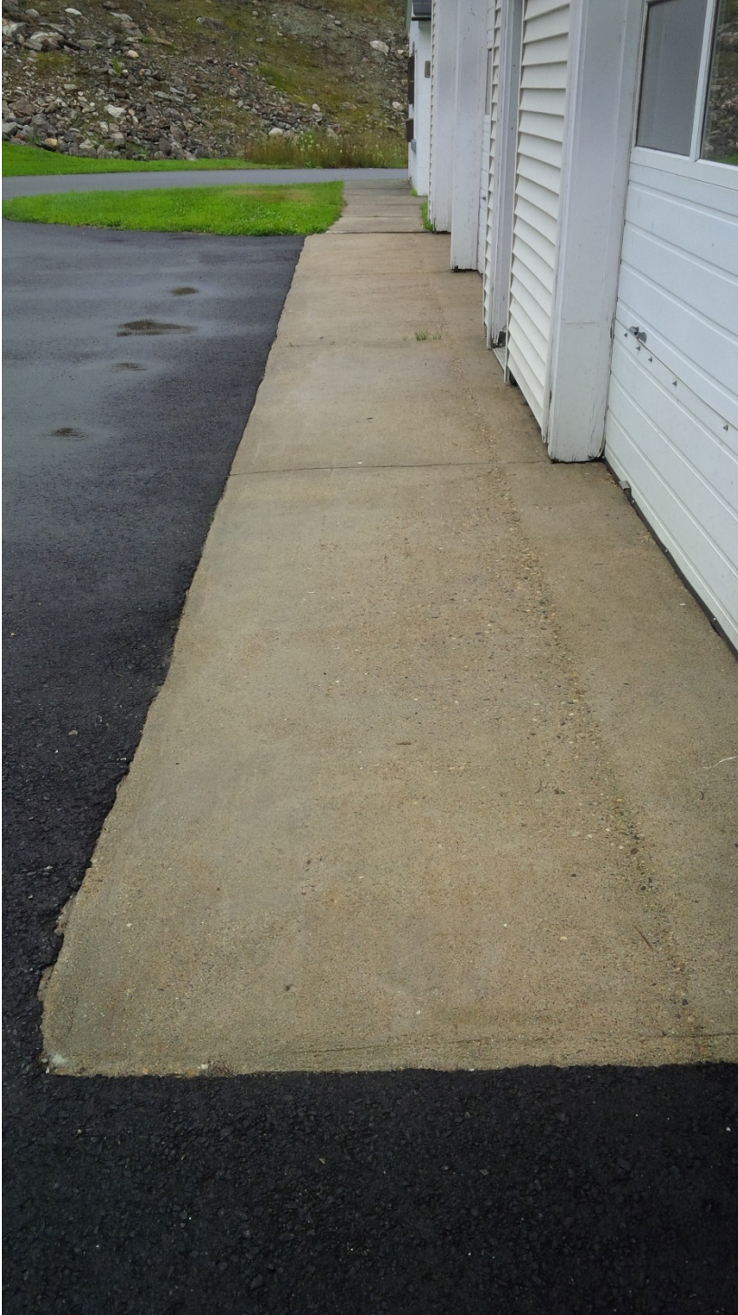
Informational Photo Number 5: Otter Brook Lake – Current condition of apron
