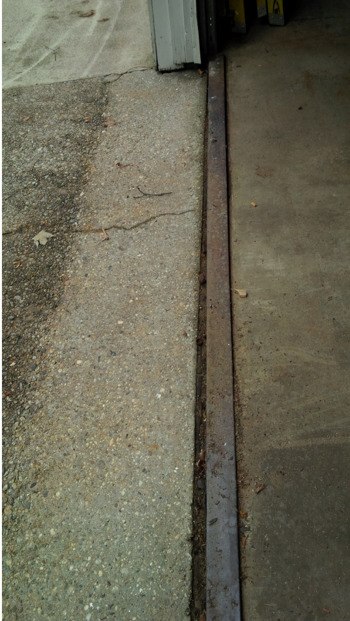
Informational Photo Number 3: Surry Mountain Lake – Current condition of apron
