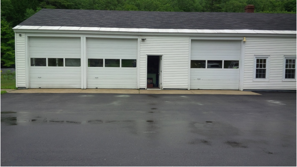
Informational Photo Number 4: Otter Brook Lake – Current condition of apron
