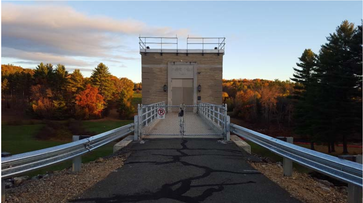
Informational Photo No 3: View looking North at the Gate House from the dam roadway.
