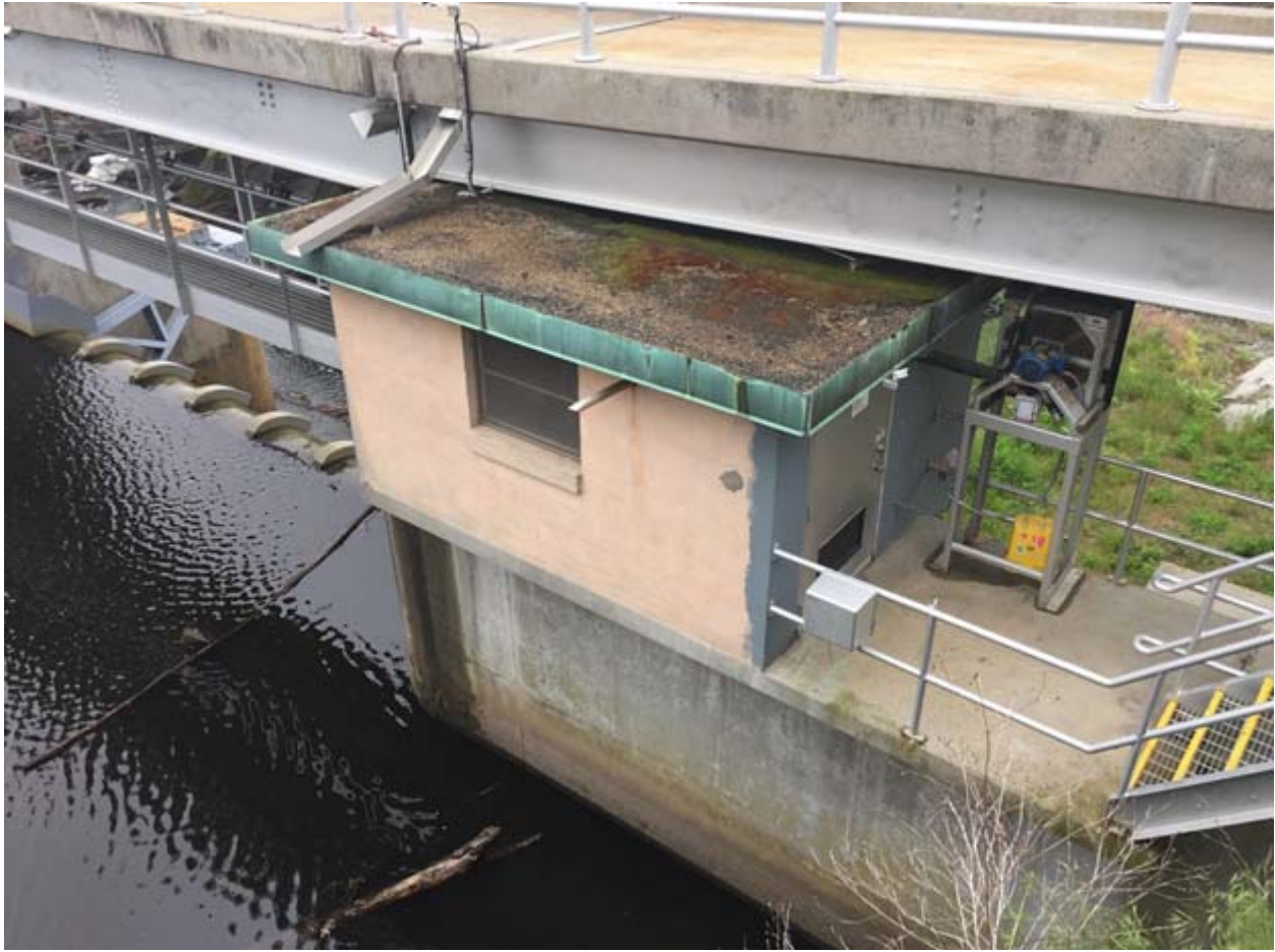
Informational Photo No. 4: View of Woonsocket Falls Dam, window (1) to be replaced and one of the two (2), single exterior doors to be replaced.
