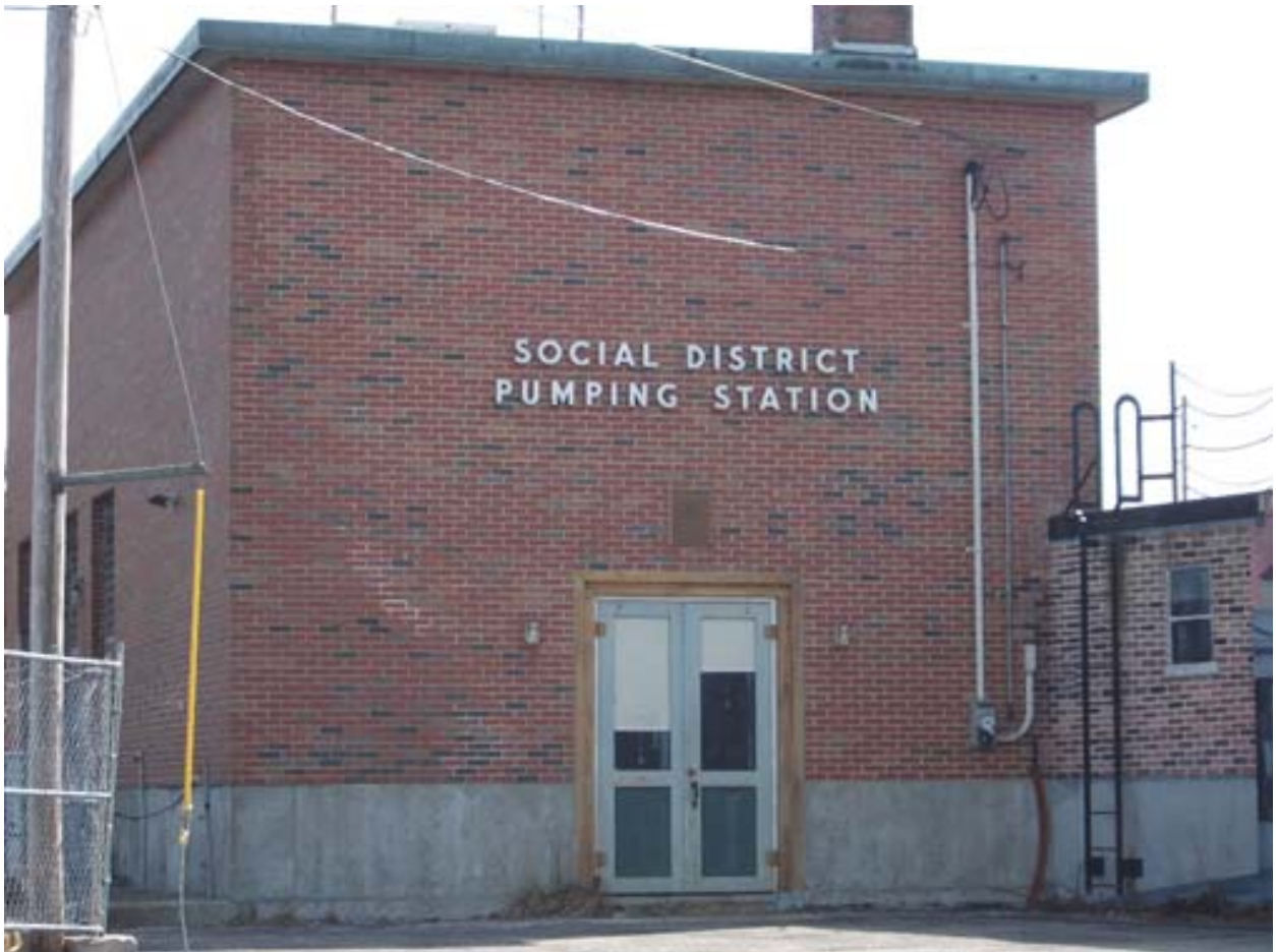
Informational Photo No. 2: Social District Pumping Station existing exterior double door. Door at Hamlet District Pumping Station is similar.
