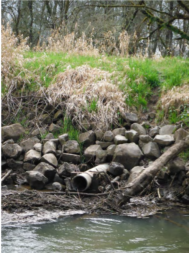
Outlet fish egress pipe at Ruby Water Control Structure looking south. Photo was taken at 10:20am on 3.28.2013 during an outgoing tide. Water stage was approximately 8.75 NAVD88 and the low tide for the day was 3 hours after this photo was taken.
