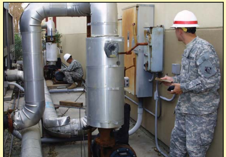
Soldiers with the 249th Engineer Battalion check the electrical requirements for an air conditioning unit at the Island Community Center in Galveston, Texas in September 2008, soon after Hurricane Ike struck the area. Soldiers from the 249th continue to respond to disasters when called upon. (Photo by Brooks O. Hubbard IV, Los Angeles District)
