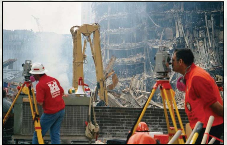
Corps of Engineers structural experts kept a constant watch on the heavily damaged structures surrounding Ground Zero, to look for any signs they might collapse while recovery efforts were taking place. (File Photo)
