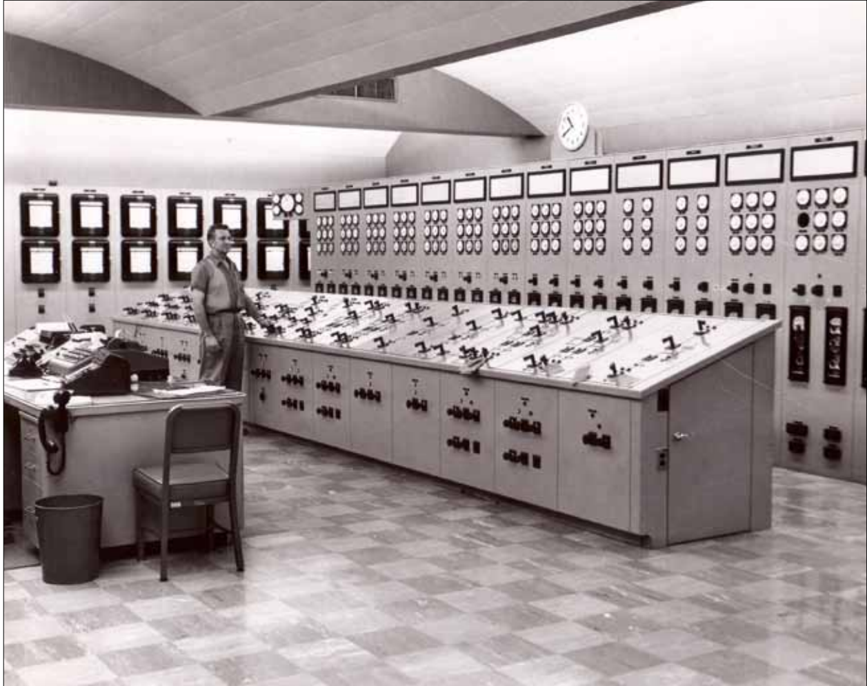
Clarks Hill (Thurmond) Powerhouse Control Room, 1955 (USACE photo).
