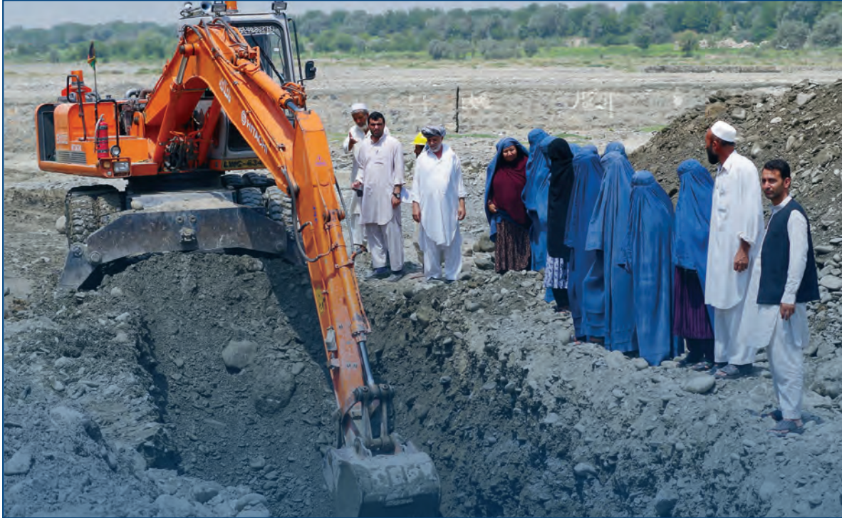
Mando Zayi District Development Assembly leaders from Logar Province, Afghanistan, conduct a monitoring visit of a USAID-funded project to build a wall to shield farmland from flash floods. Photo: USAID/Ahmad Salarzai (November 12, 2013)
