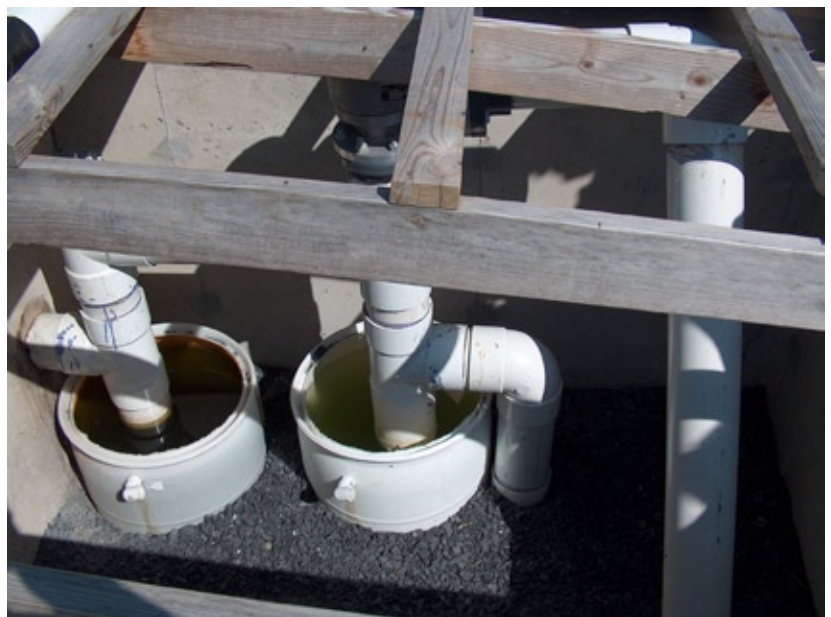
Drip pots that remove water droplets and act as over pressure relief valves set at 1.5 inches of water column pressure
