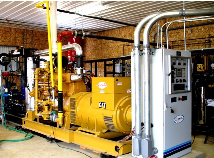
Combined Heat and Power Unit (CHP)
