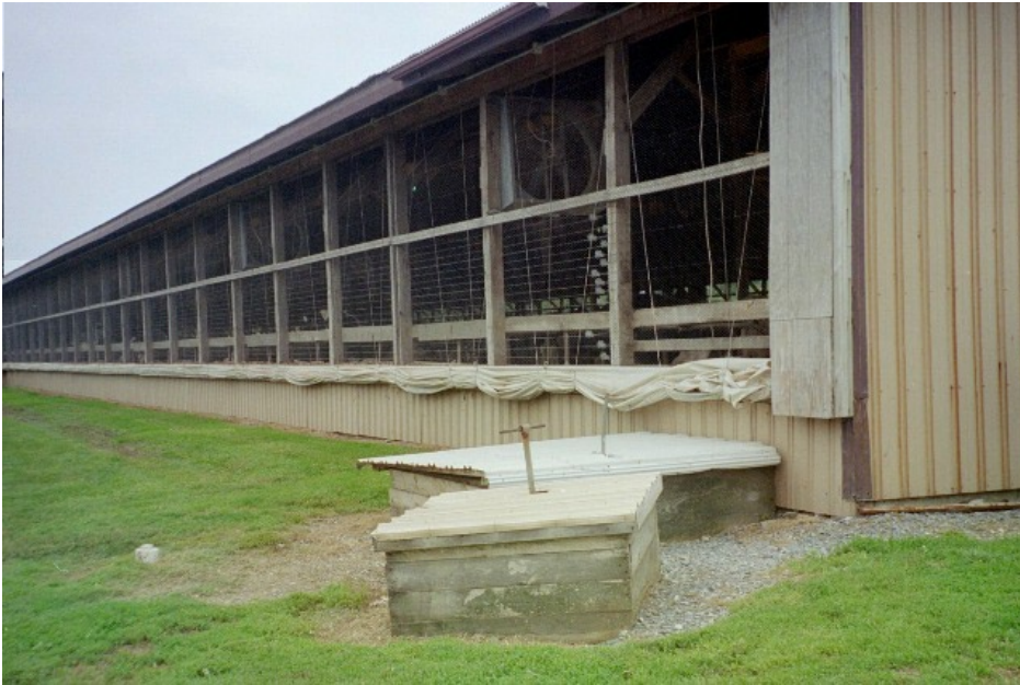
Manually valved pits for directing raw manure to the digester or to the storage lagoon
