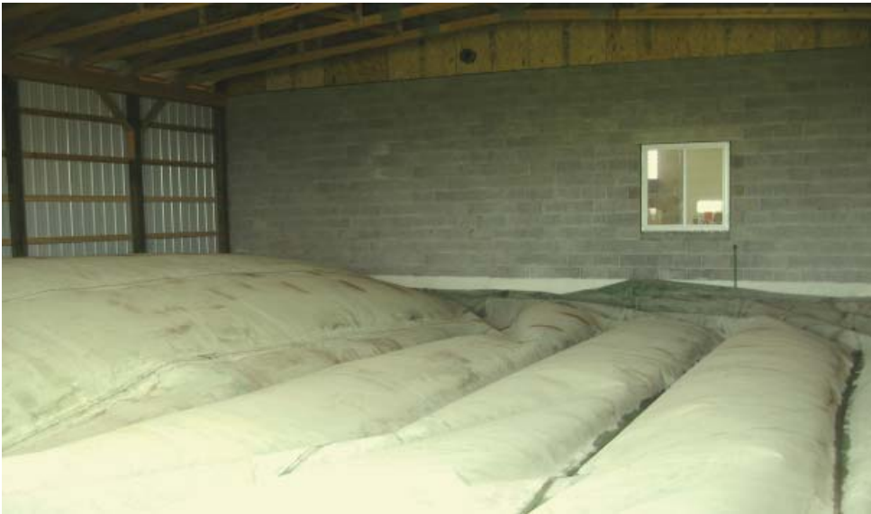
Biogas Storage, bag volume 15,120 ft 3 , Bladder Building 40'L x 45'W
