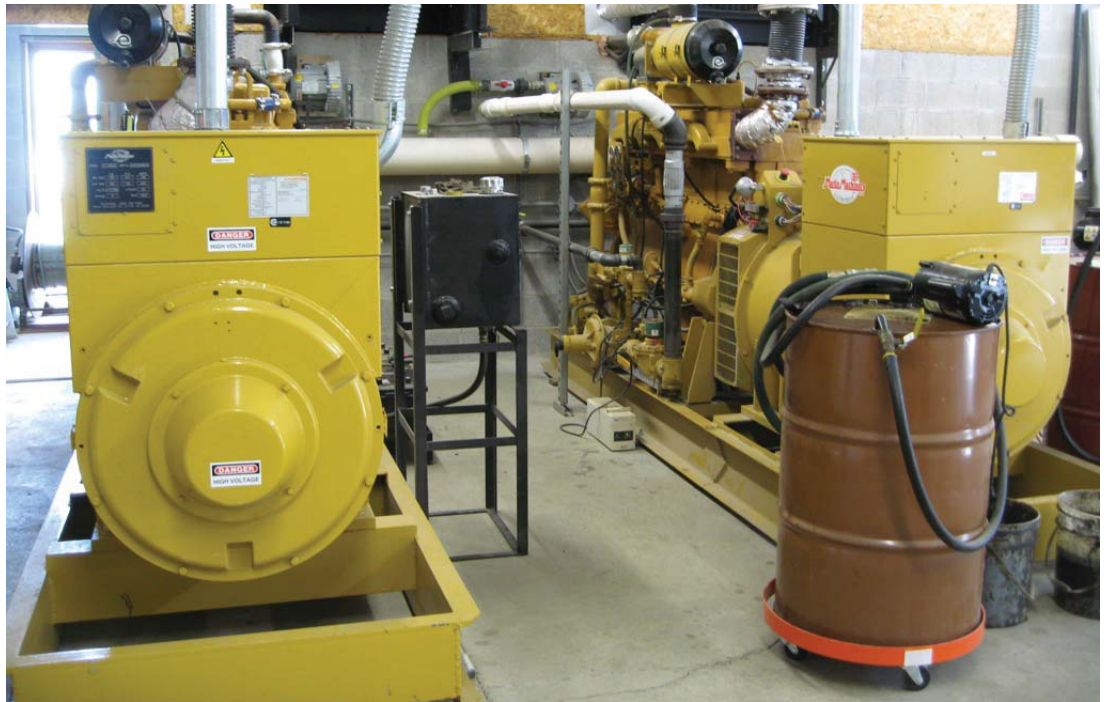
2 - G342NA Caterpillar engines with 3 phase 130kW generators
