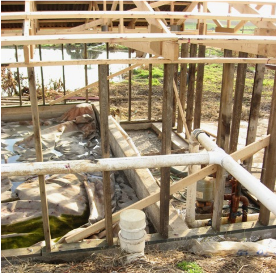
Partial view of the digester, construction of the new roof and the storage pond in the background.
