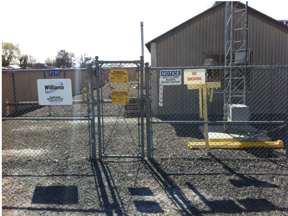
Figure 8.2: Example meter station in Sunnyside (9390 Emerald Road)
