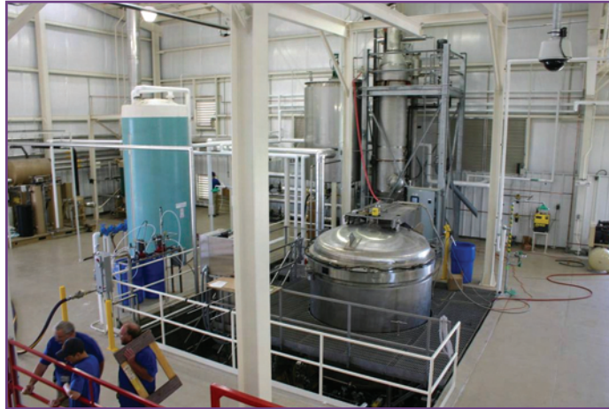
Figure 1. A tissue digester in a fixed alkaline hydrolysis facility. (Photo courtesy of Waste Reduction by Waste Reduction, Inc., Indianapolis, IN)
