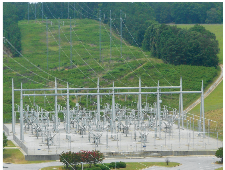
GA-AL-SC System Customers approved nearly $2 million to install eleven 230,000 volt circuit breakers in the Richard B. Russell switchyard reliably tying the plant to Santee Cooper and Southern Company transmission lines. These new Sulfur Hexafluoride Gas circuit breakers have eliminated the need to store and transfer insulating oil in close proximity to downstream ecosystems. Photo:USACE
