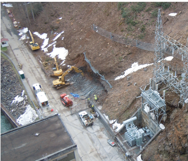
Excavation begins on a new station circuit breaker building beside the entrance road to Philpott powerplant. Moving the generator breakers from the control room will eliminate arc flash personnel hazards and improve maintenance access. In the right foreground, the new step-up power transformer was placed in service in 2014. Photo:USACE
