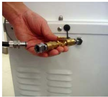
Exhibit 14: Pump shutoff valve connection.
