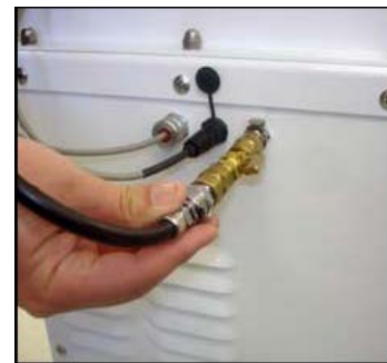
Exhibit 15: Connection of air line to pump shutoff valve.
