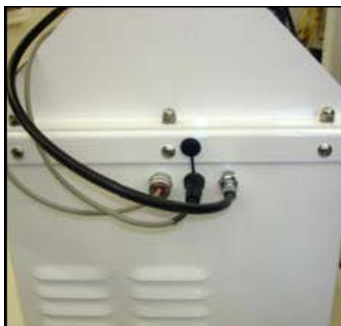
Exhibit 13: Vacuum (air) line disconnect.
