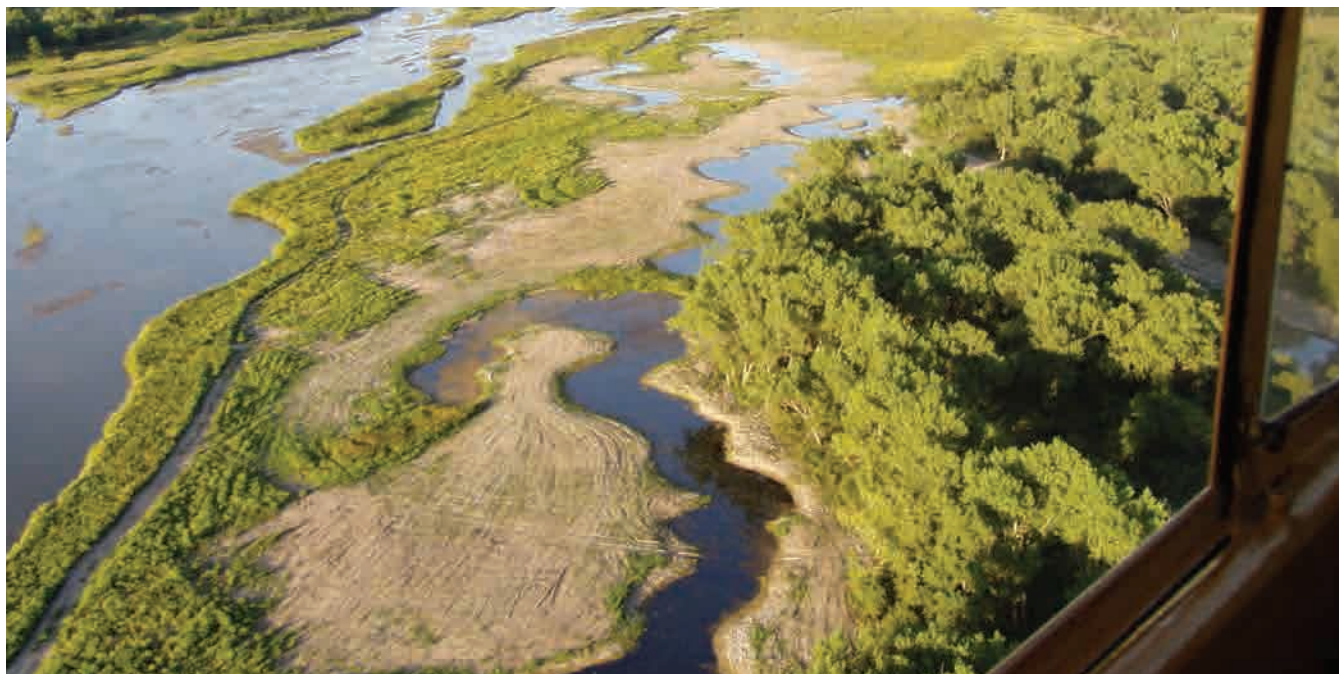
Central Platte Riverine wetland restoration project located in Hall County, Nebraska. Photo by Shawn Harder of Harder Dozer and Scraper, contractor for project.
