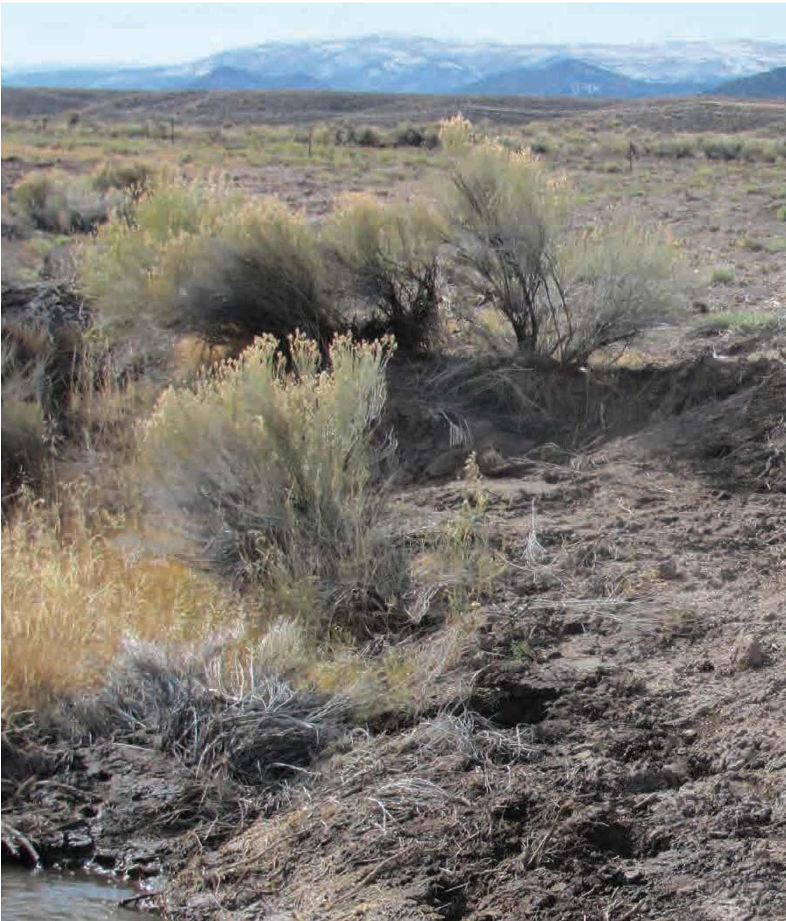
Utah PFW staff re-seeding a riparian area immediately after heavy equipment restoration work. USFWS photo.
