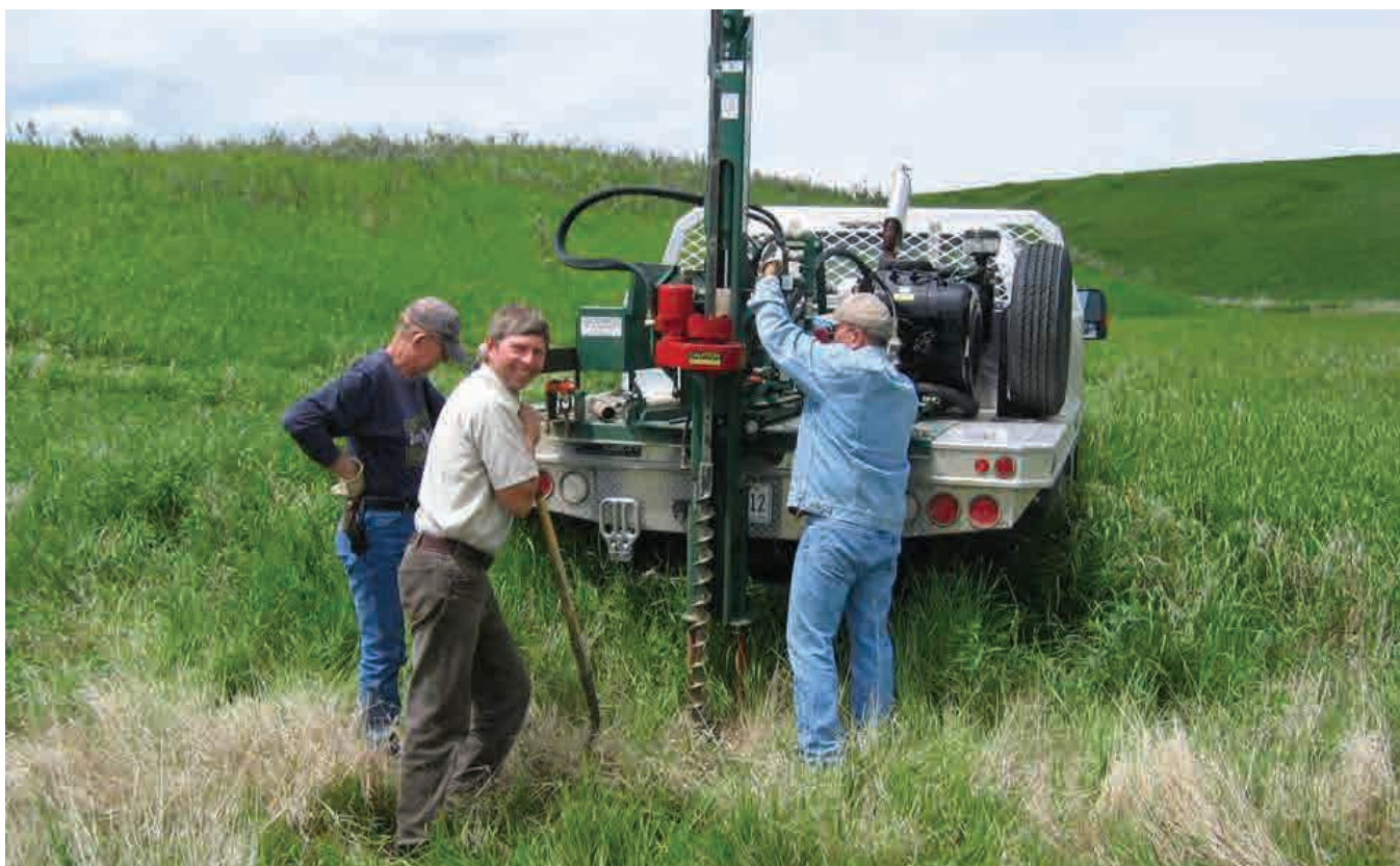
ND PFW Biologist gets assistance from NRCS Soil Scientists and their soil sampling truck to determine whether a site has suitable material for dam construction on a PFW wetland creation project. USFWS Photo.
