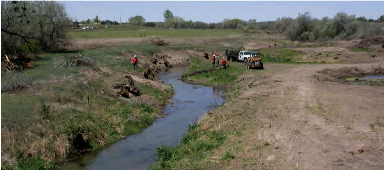
Contractors restoring the natural form and function of a prairie stream section. Photo by Matt Filsinger, USFWS.
