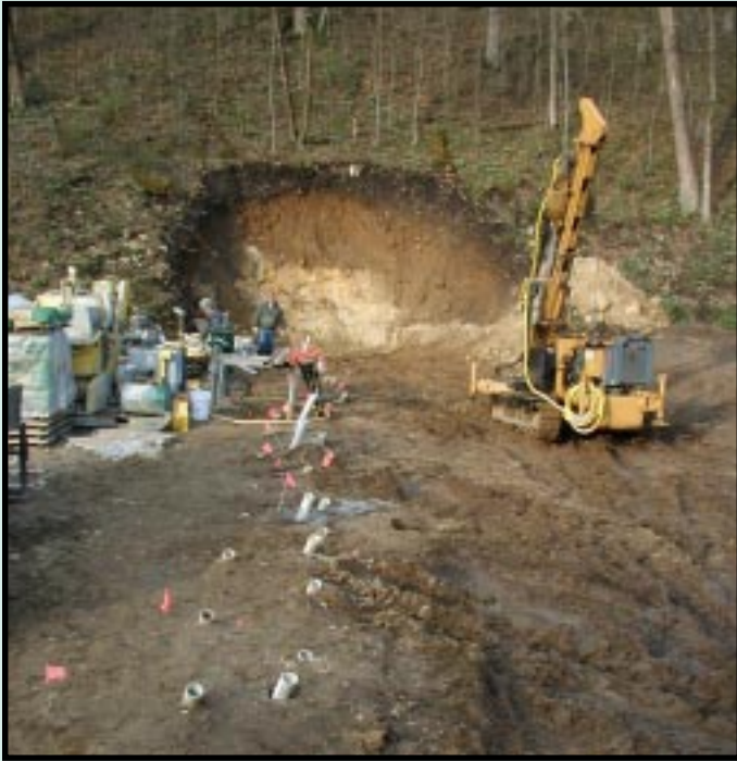
Grout, a mixture of cement, water and clay, is injected through boreholes into voids in the rock. The grout curtain reduces water flow through rock in the dam foundation.
