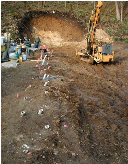
Grout is injected through boreholes to slow water movement beneath and around the dam.
