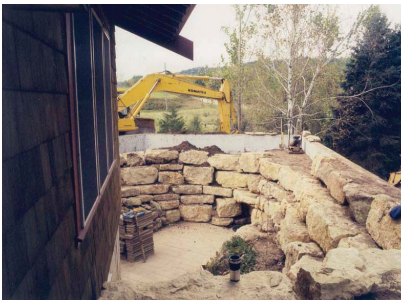
Flood wall installed to protect home in case of dam breach.
