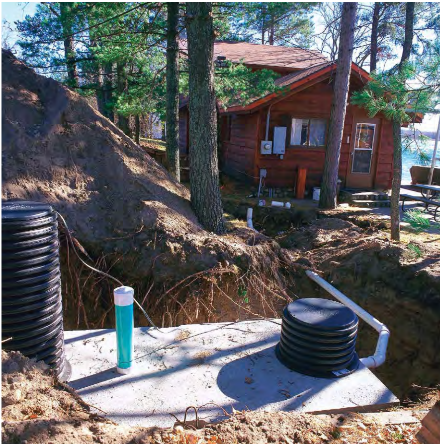
A newly installed septic tank at a lake-side cabin. The tank has been installed in a hillside, which requires tall and short access points to facilitate periodic inspection and maintenance and accommodate slope.
