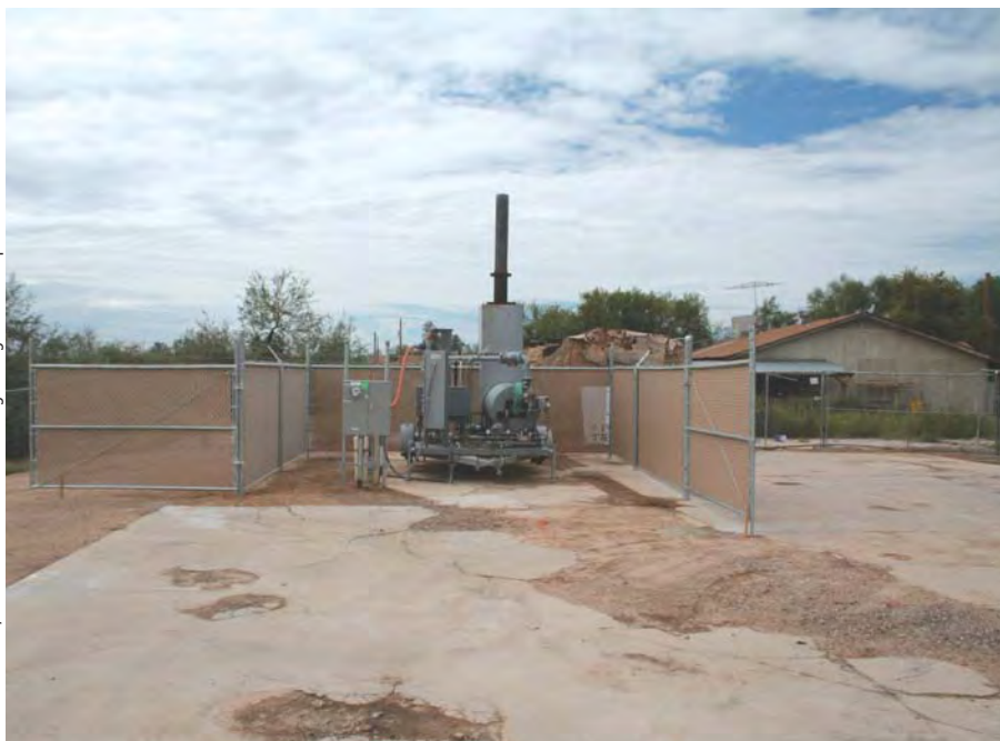
Arizona's Gila River Indian Community, along with USEPA, installed and activated this LUST site cleanup system to remediate hydrocarbon-contaminated soil and ground water. In what is expected to culminate in a 10-year cleanup effort, the final price tag may exceed $2 million.
