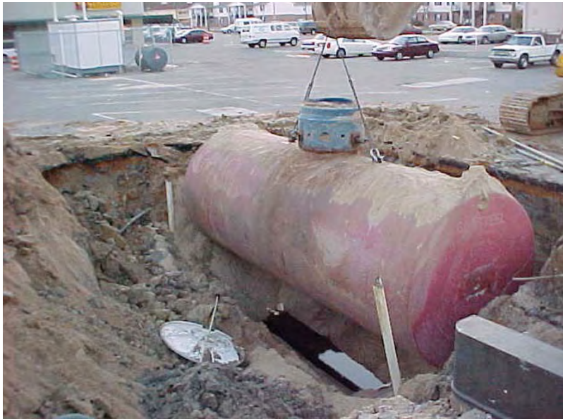
As a UST is removed, gasoline released from the UST system becomes apparent in the tank pit. Discovering the contamination is only the beginning of a long and expensive process that includes site investigation, cleanup, monitoring, and often litigation.
