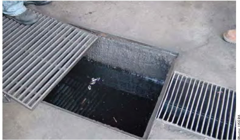
Existing motor vehicle waste disposal wells like the one in this photo can provide a direct contaminant pathway to ground water.
