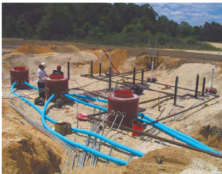
A new UST system is being installed. Leak prevention depends on the proper installation of a UST system that meets regulatory standards. This system must then be properly operated and maintained.
