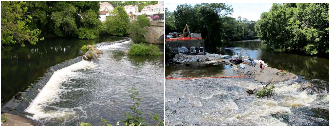
The Pawtuxet River Falls prior to the dam removal (left) and during the dam removal where excavators remove the concrete spillway (right).
