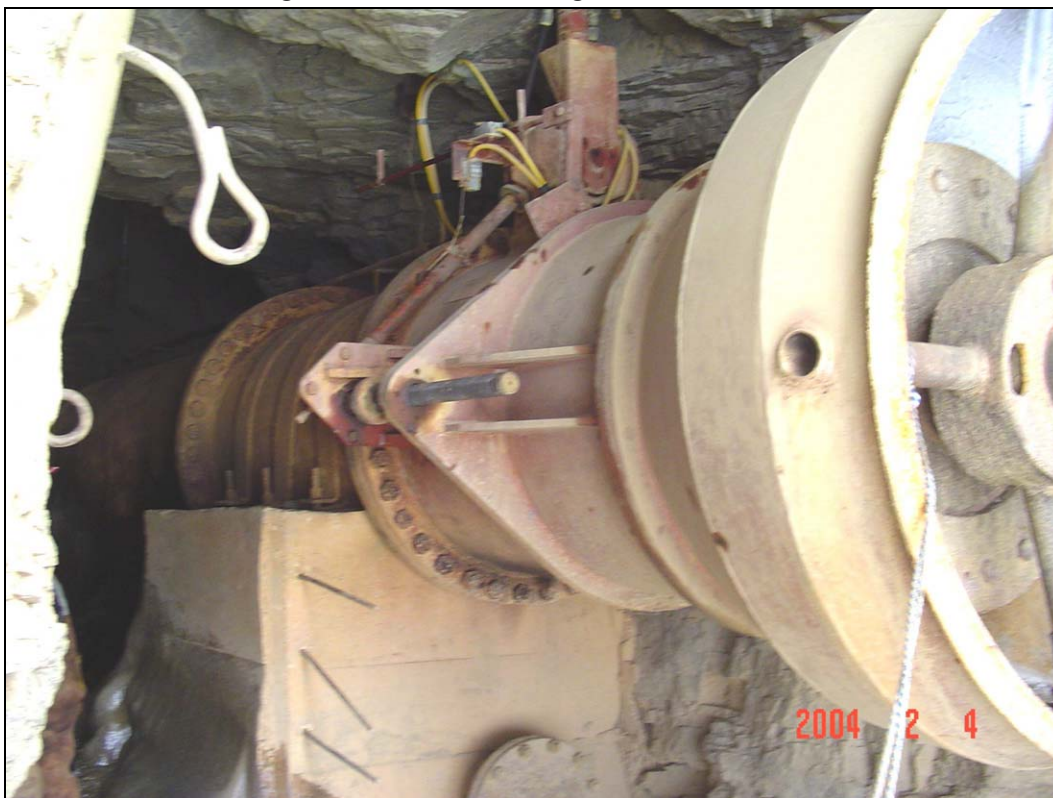
Figure 2-89. Howell-Bunger Valve at Outlet
