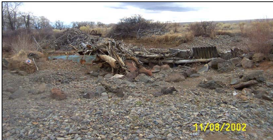
Figure 2-105. Poor River Condition– San Jose Ditch No. 1
