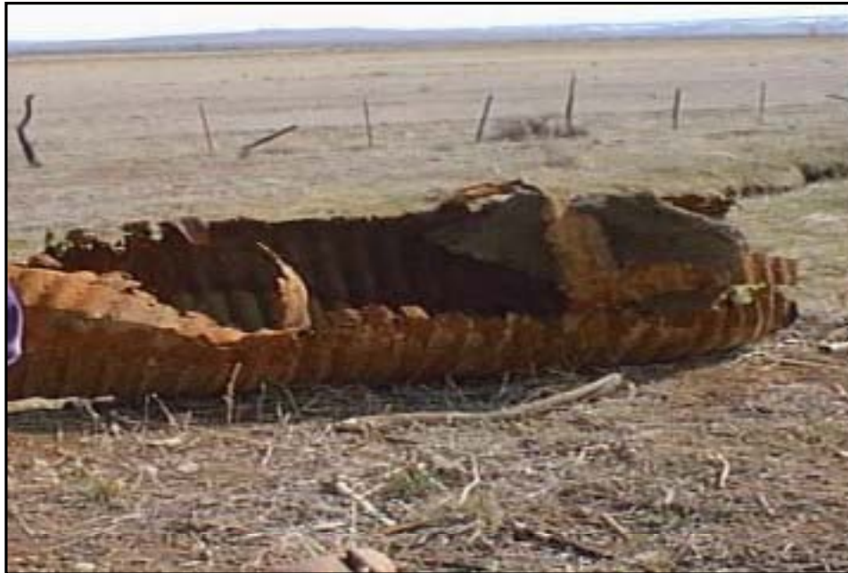
Figure 2-108. Photo of damage to culvert after exposure to Alamosa River Water
