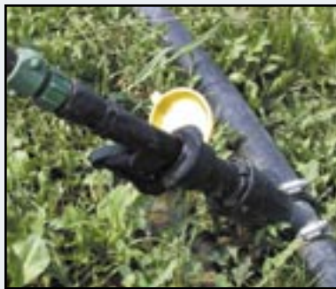
Quick coupler hydrants are used on this one inch water line.
