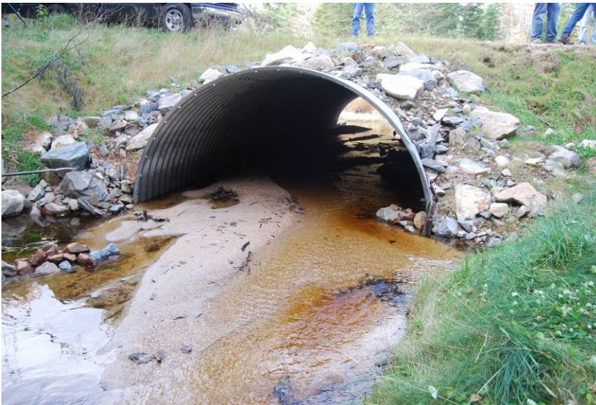
Figure 2. Stream connectivity restored at road/stream crossing by replacing traditional round culvert with open-bottom arch culvert.
