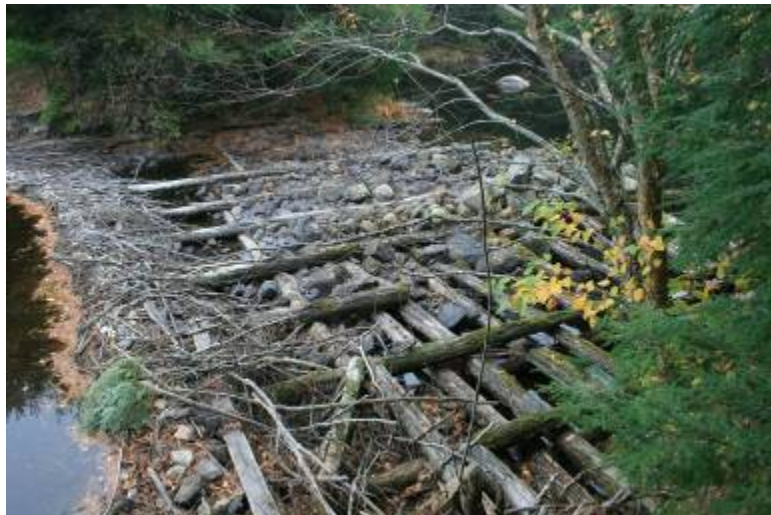
Figure 9. Remnant Dam at the outlet of Fourth Machias Lake. This structure is not in the State or National Dam Database. Picture is looking north across river. (Oct 2007) Photo by Scott Craig
