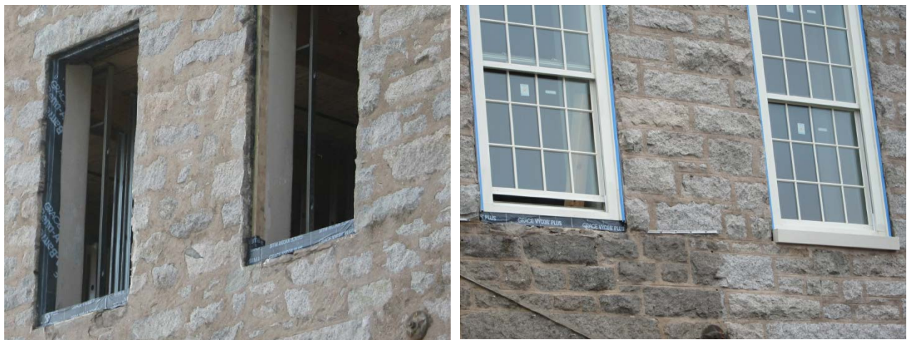
Figure 45. Left: Membrane flashing wrapping window opening; Right: Exterior view of window assembly and completed unit
