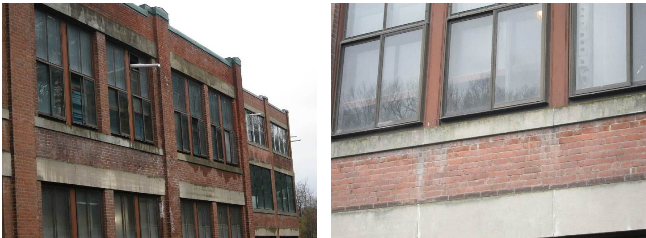
Figure 29. Improper drainage off window faces, and staining at window sill grout joints
