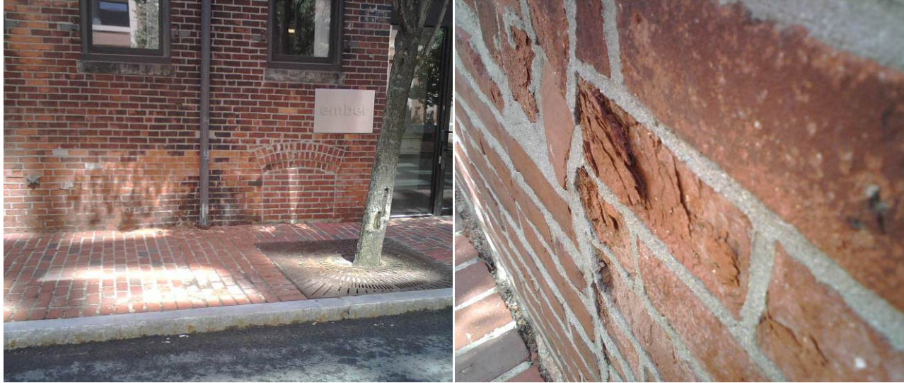
Figure 65. Left: FT damage at downspout disconnection; Right: delamination of brick
