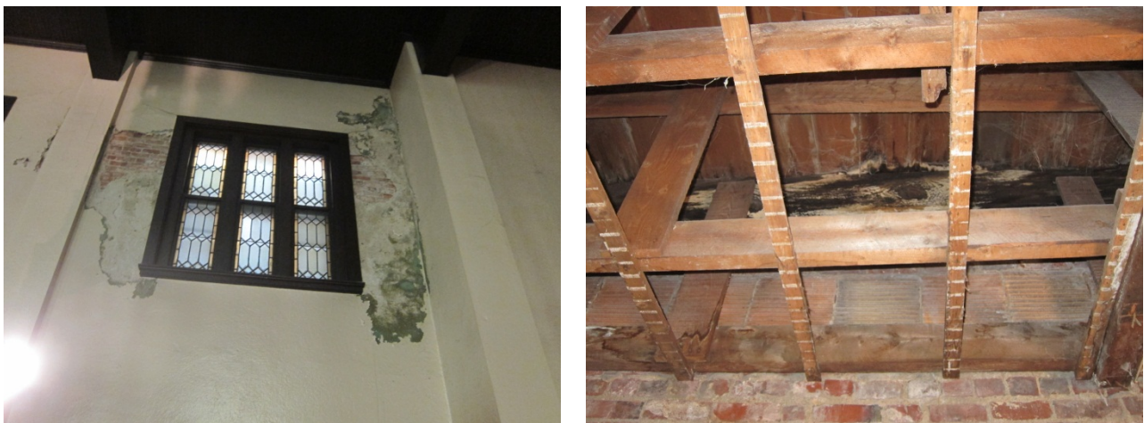
Figure 84. Interior details showing previous moisture issues at window and roof-wall interface
