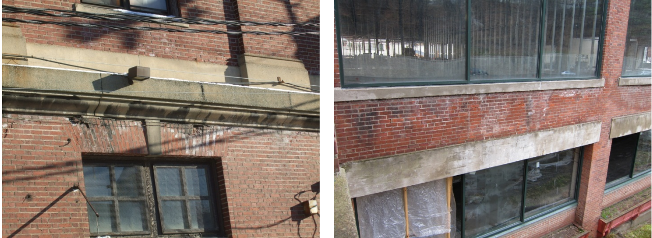
Figure 83. Exterior details that demonstrate FT damage in existing masonry buildings
