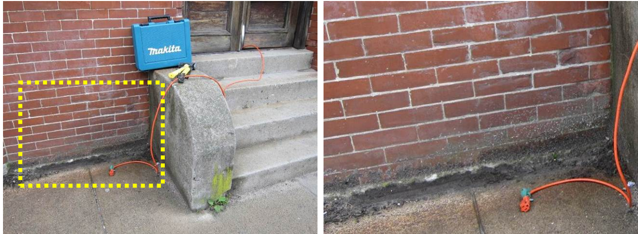
Figure 75. Brick condition adjacent to front steps, splashback evident
