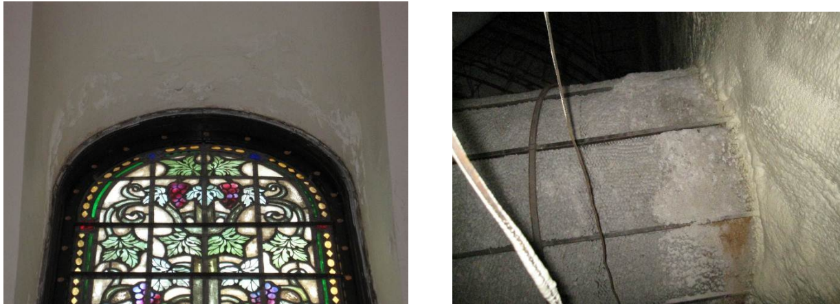
Figure 58. Moisture issues at chapel windows
