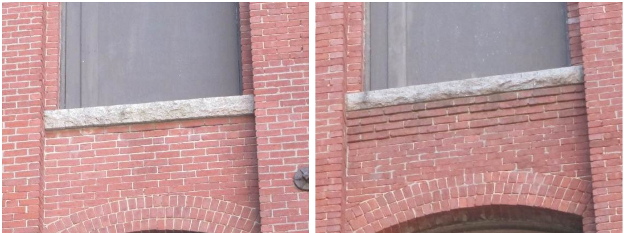
Figure 37. Left: Window sill without brick corbeling (left); Right: Window sill with brick corbeling, showing different mortar erosion patterns
