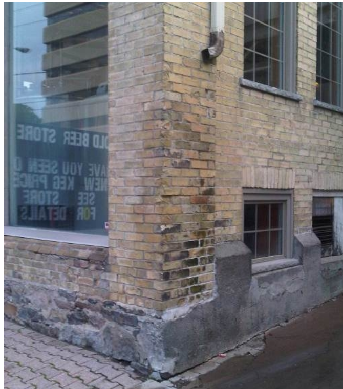
Figure 66. Disconnected downspout and related damage to masonry
