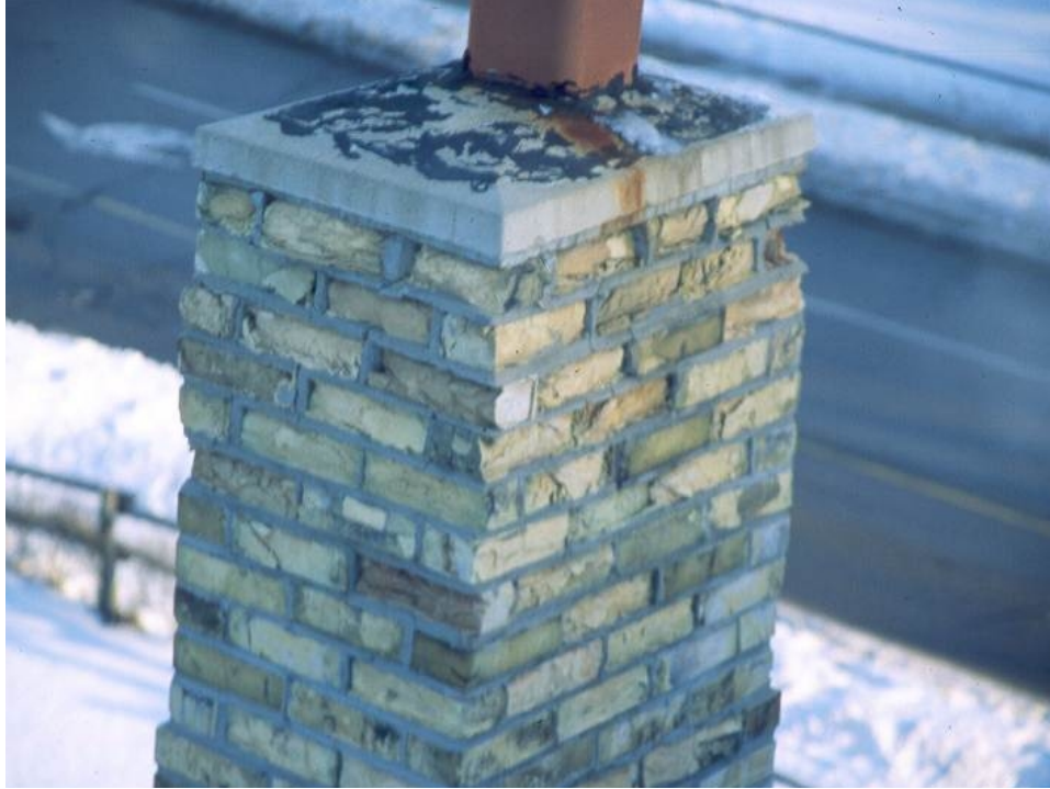
Figure 59. Severe FT damage at existing chimney; lack of projecting cap with drip edge
