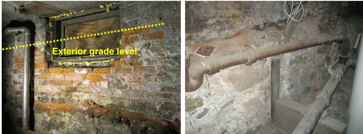
Figure 69. Left: Severe subfluorescence and spalling at basement window; Right: Stone shelf below grade
