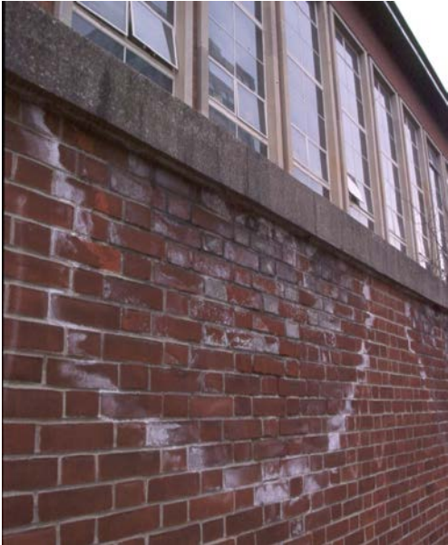
Figure 35. Failed mortar joint at sill from concentrated runoff, resulting in brick failure
