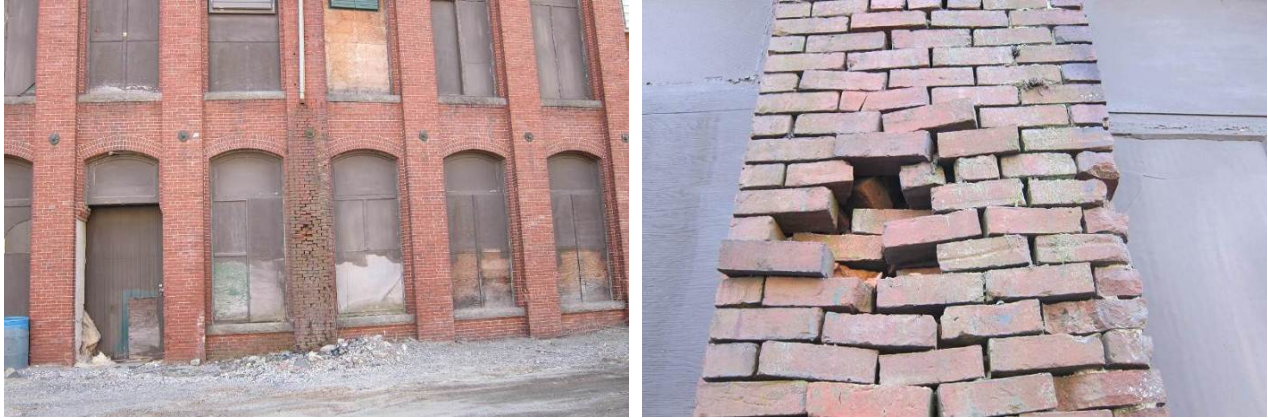
Figure 67. Left: Damaged pilaster at downspout; Right: Severe mortar erosion
