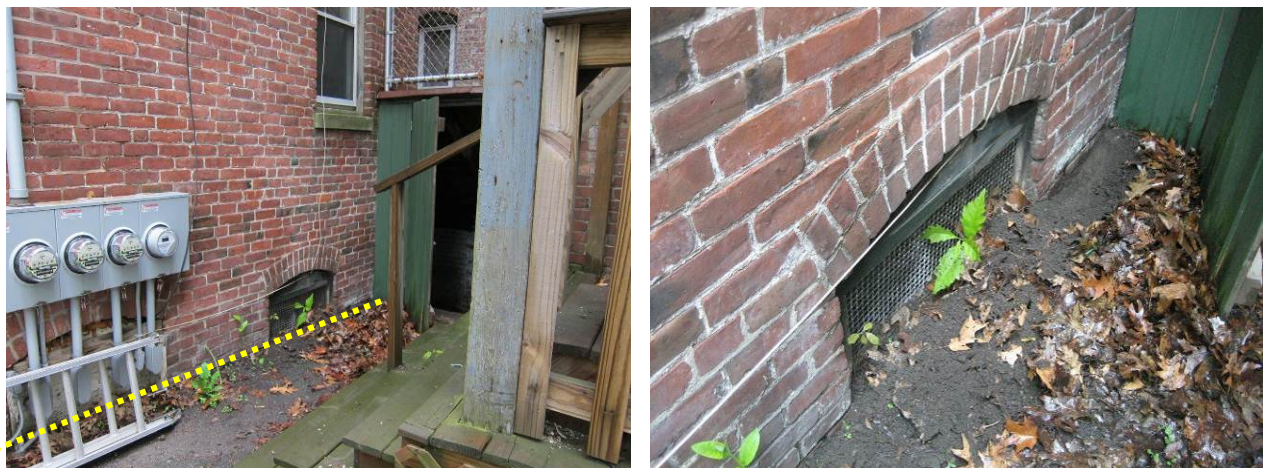
Figure 70. Left: Rear wall near subfluorescence damage visible in basement; Right: Buried window
