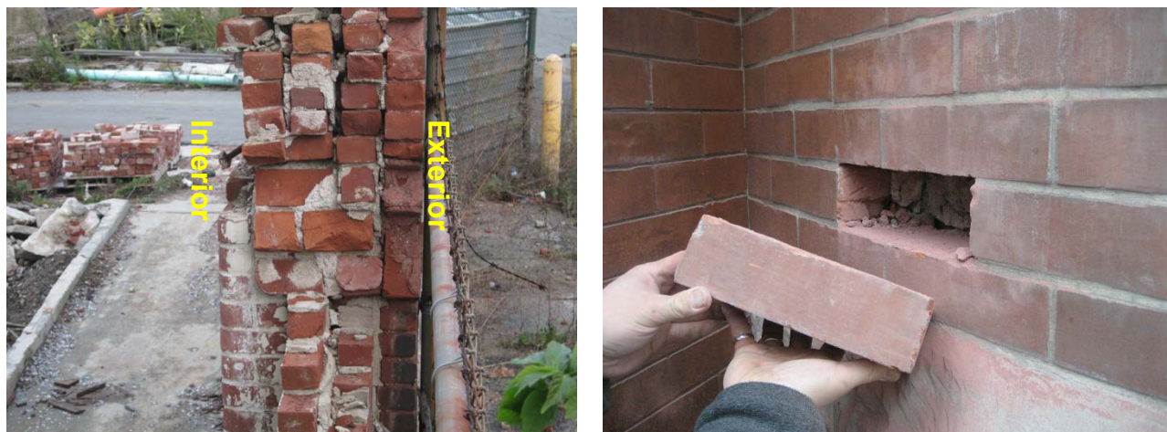
Figure 14. Voids commonly found between wythes of brick in masonry walls
