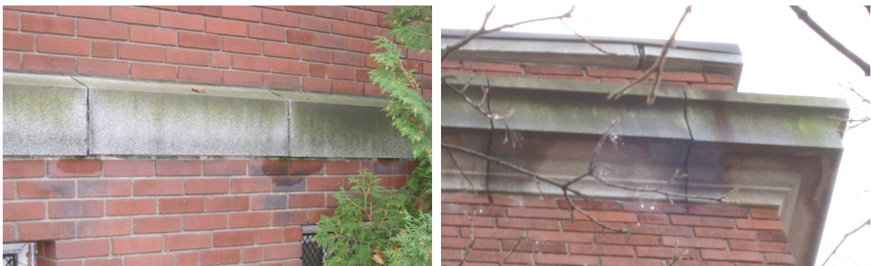
Figure 51. Water concentration at stone belt and cornice joints
