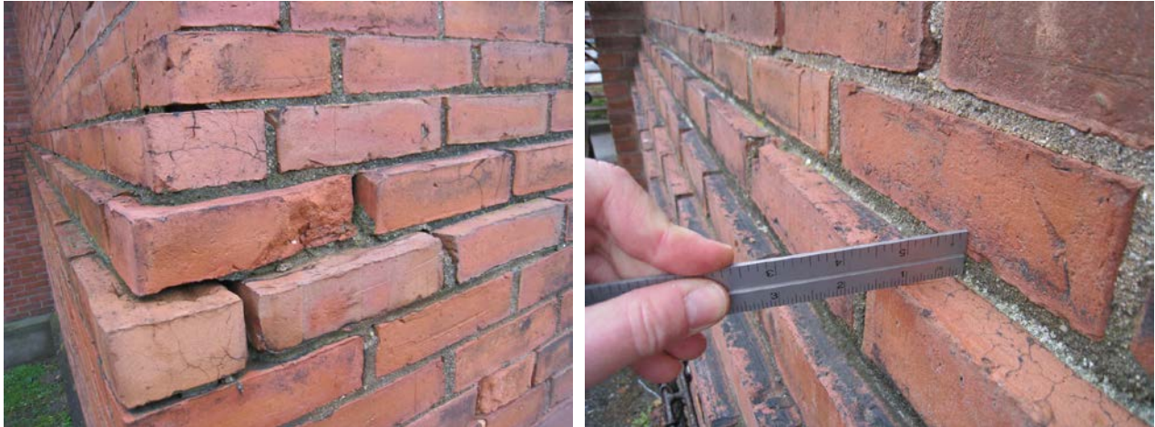
Figure 50. Steps in brickwork, and related cracking/FT damage
