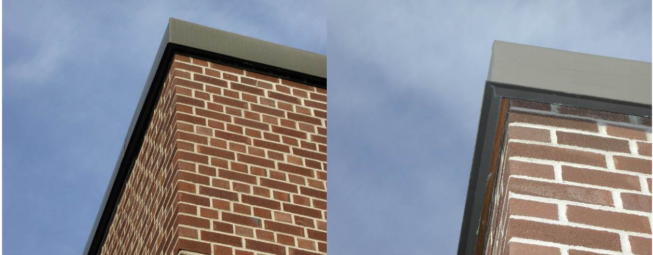
Figure 62. Improved drip edge overhang at coping
