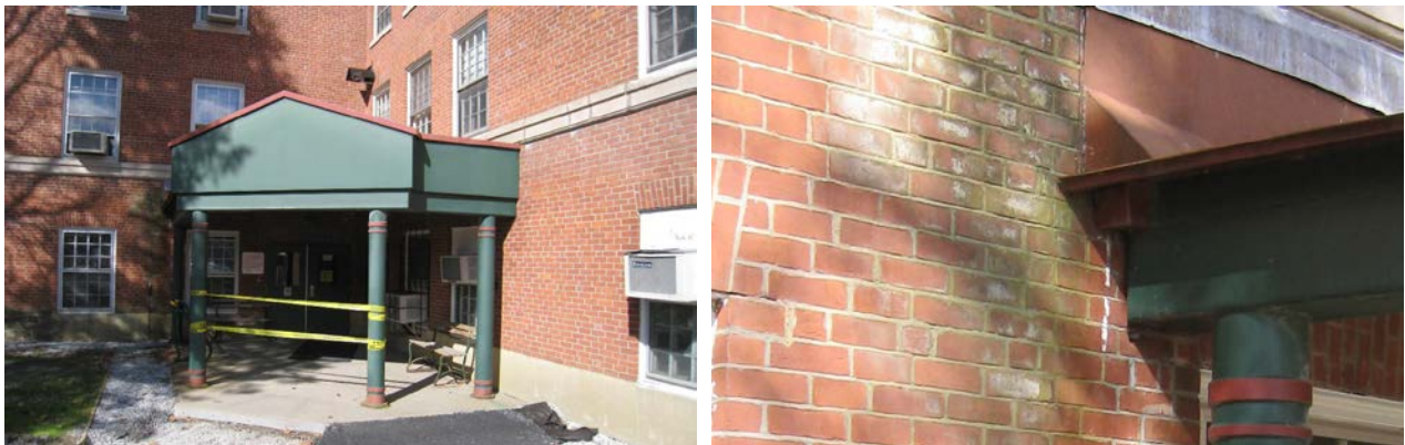
Figure 53. Left: Retrofit roof over entrance; Right: Water runoff concentration at roof-wall interface
