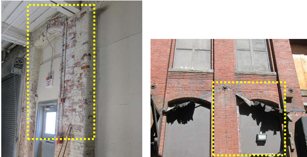
Figure 56. Left: Interior paint/parging delamination; Right: Exterior conditions for comparison
