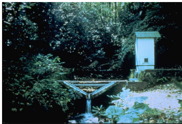
Figure 36: Flow measuring include portable instruments and fixed devices such as weirs and flumes. As illustrated in the above photo, a weir and water level recorder can provide measurements for a wide range of flows.
