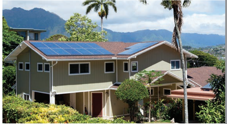
SolarCity's work with NREL at the ESIF to optimize PV inverter technology will ultimately enable greater deployment of solar PV on homes and buildings across the country. Photo from SolarCity
