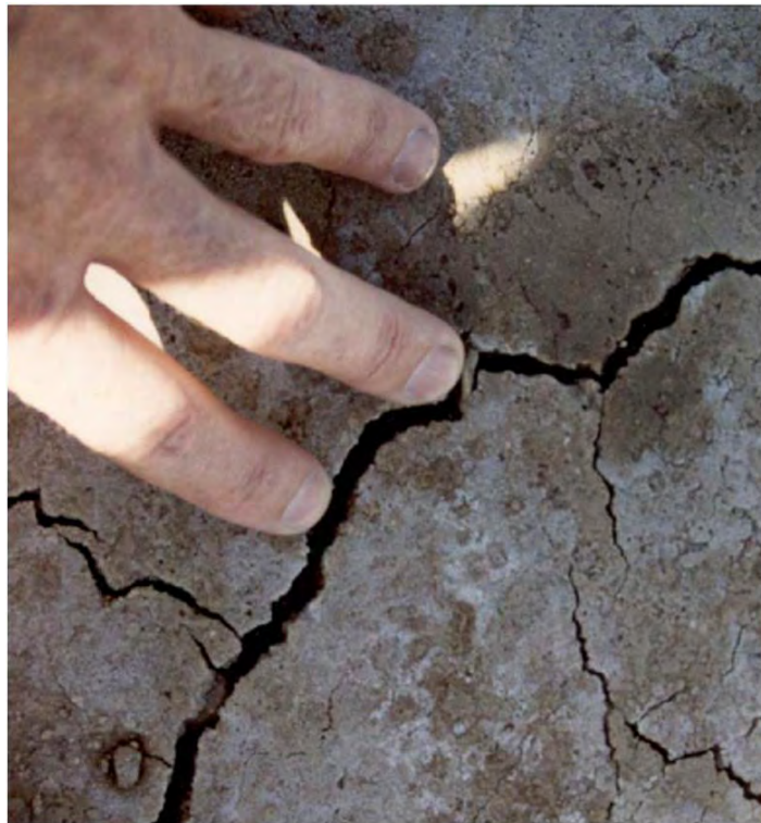
Figure 7. Desiccation Cracking in Clay Barrier Layer
