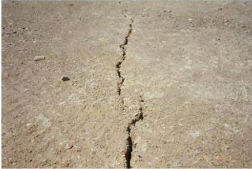
Figure B-2. Surface Crack in Brittle Cover Soil
