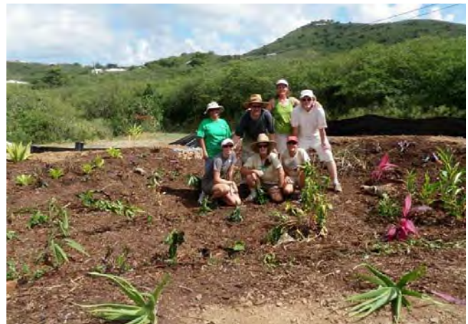
Project partners and volunteers installed a demonstration rain garden at a residence in Hope & Carton Hill, St. Croix, USVI (October 2012).
