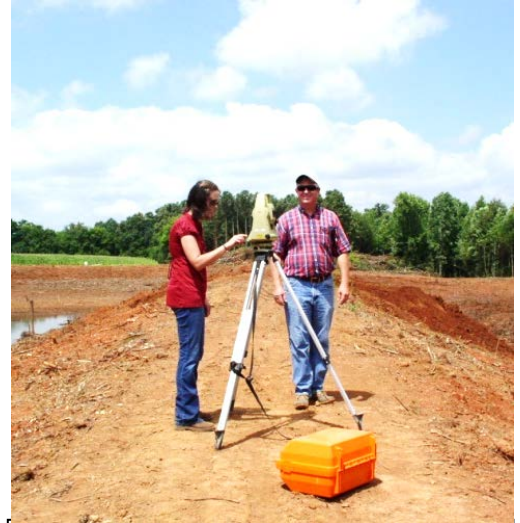
(l-r) Hannah South (Civil Engineering Student) receives training from Tim Williams (Resource Engineer) on the use of the total station to survey the 10 acres.
