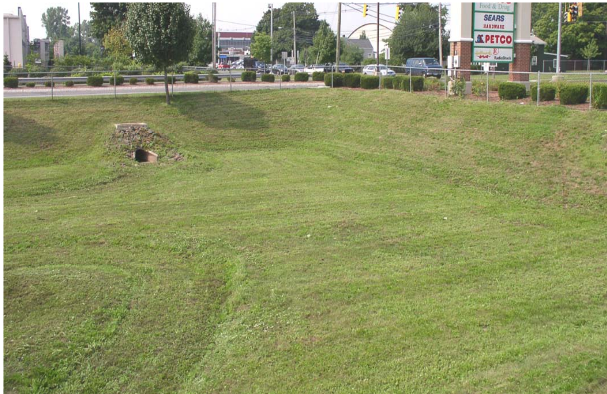
Fig. #4 Dry Detention Basin Photo Credit: Tom Ladny, NRCS
