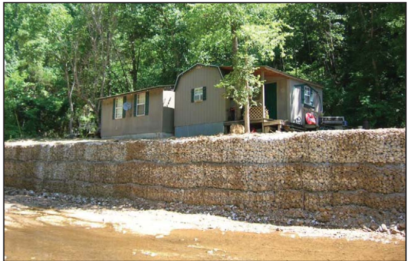
After: Gabion baskets protect Deanna Young's home and stabilize the bank along Adds Creek.
