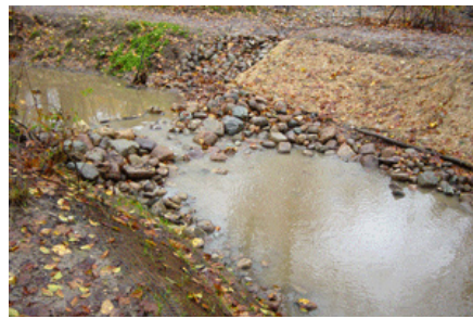
Many techniques are used to restore streams. Above, a newly installed rock riffle will slow stream flow and protect the creek from erosion. photo: http://waldendesign.net
