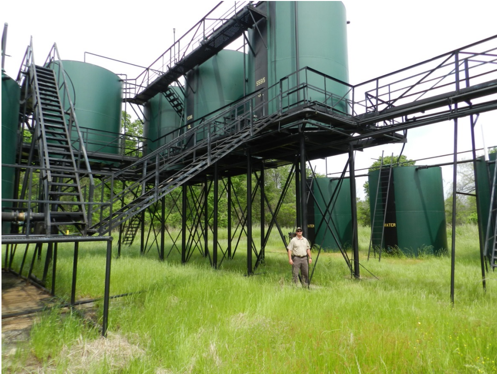
Figure A2-6. Oil production facility elevated above floodplain at Catahoula NWR, LA. P Ramirez/FWS Photo
