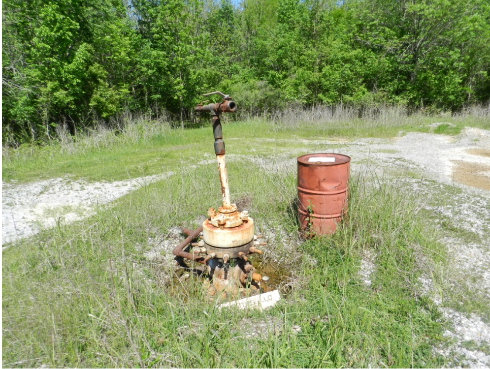
Figure A2-4. Inactive well at Tensas River NWR, LA. P Ramirez/FWS Photo
