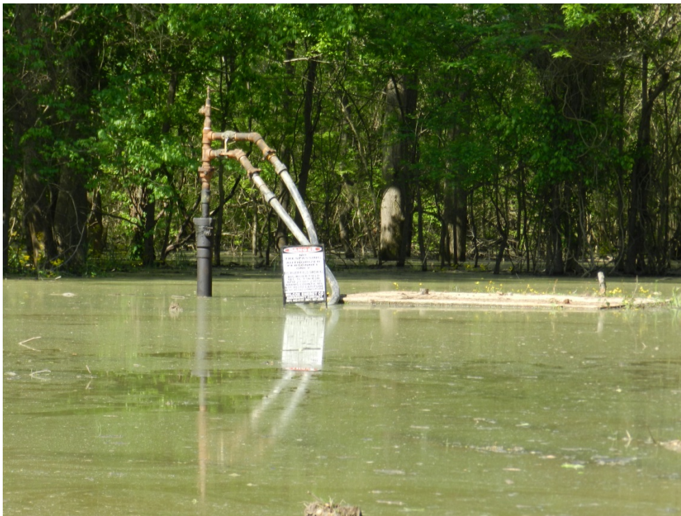
Figure A2-5. Saltwater disposal well (injection well) inundated by floodwaters at St. Catherine Creek NWR, MS. P Ramirez/FWS Photo
