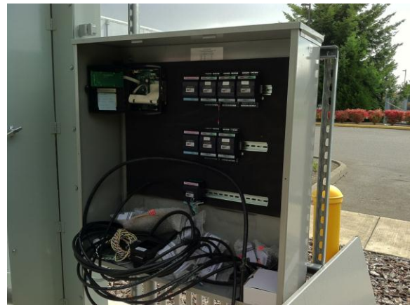
Figure IV-151: Installation of the EVSE energy management system near the Frito Lay EV parking/charging lot at Federal Way.
