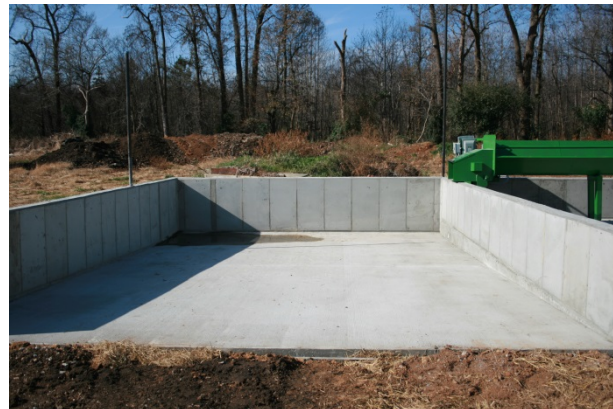
Concrete Containment Pad
