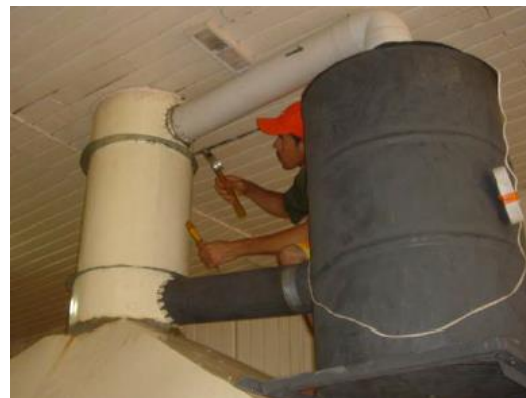
Attachment of the MCS to an existing fume hood in a small-scale gold shop.
